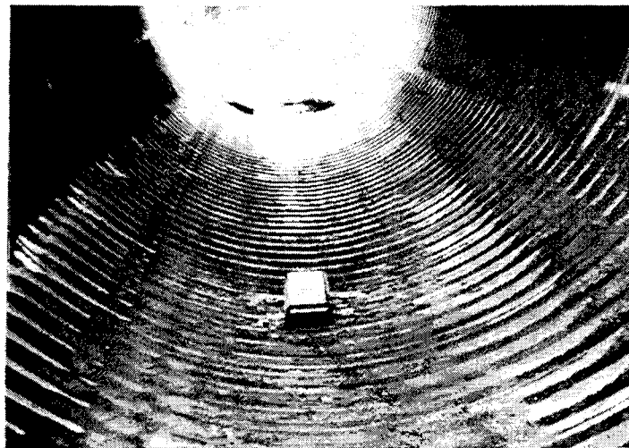
Figure 3 Internal anode attached to culvert
