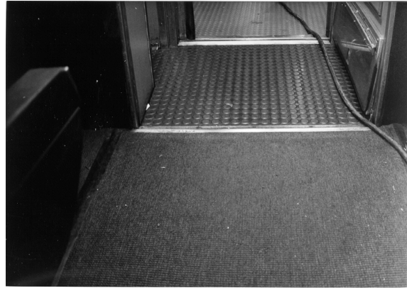
Figure 3-2. Carpet and Resilient Rubber Floor Covering
