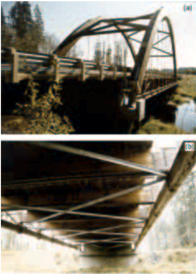
Figure 25—Cougar Smith Bridge (a) as viewed from the north showing the treated-wood arches and (b) underside of bridge showing the treated-wood deck and support beams.
