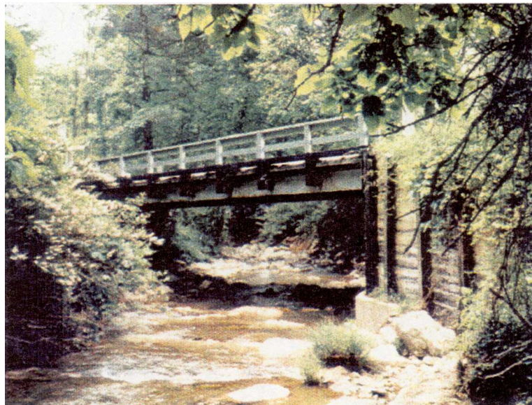
Figure 2. Valle Crucis Project (B-2179). Existing Side View (Courtesy of NCDOT Roadway Design Unit)
