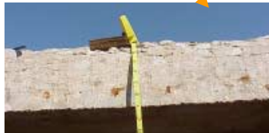
Figure A.2 Existing Damage and Crack – Beam 1
