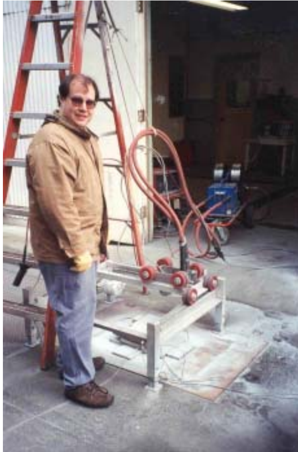
Figure 3.3: Twin-wire arc-spray equipment prior to applying TS Zn anode to concrete slab for surface temperature measurements
