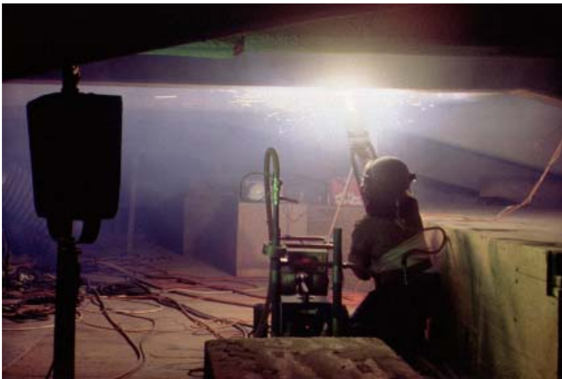
Figure 2.2: Thermal spraying Zn on a bridge substructure using the twin-wire arc-spray process
