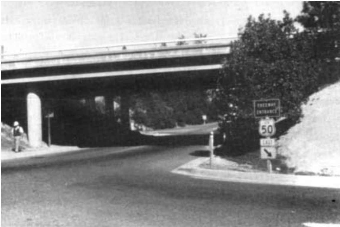
Figure 2.11: East Camino Under-crossing (CA) built in 1964 and located east of Placerville, CA
