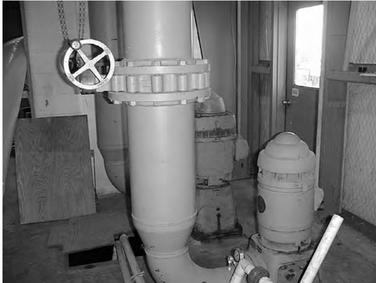
Figure 3.5: Photograph of the Inside pumps
