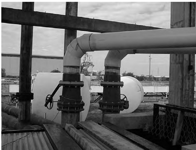
Figure 3.8: Conduits of the outside pumps (north to the right of the picture)
