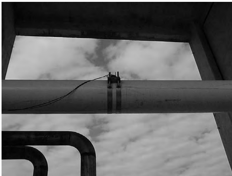
Figure 3.9: Propeller installation of the Data Industrial flow meter for the Inside pumps
