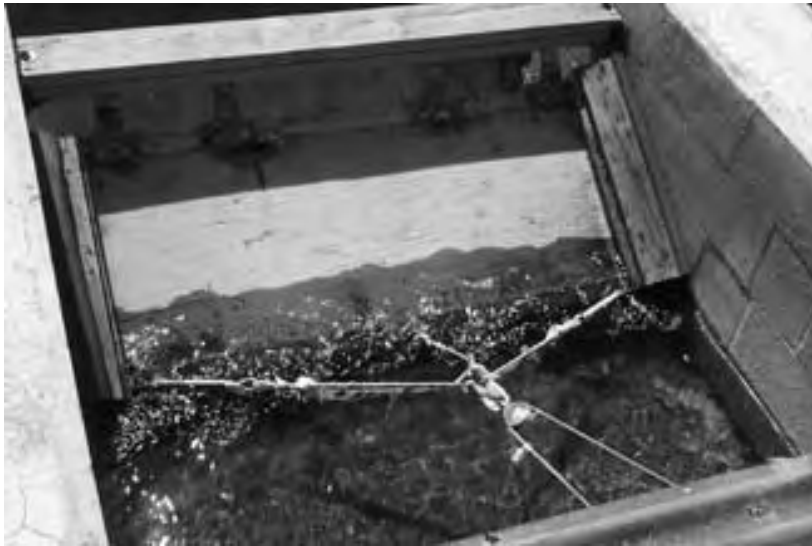
Figure 3.3: Tailgate located at the downstream end of the channel to regulate the water level
