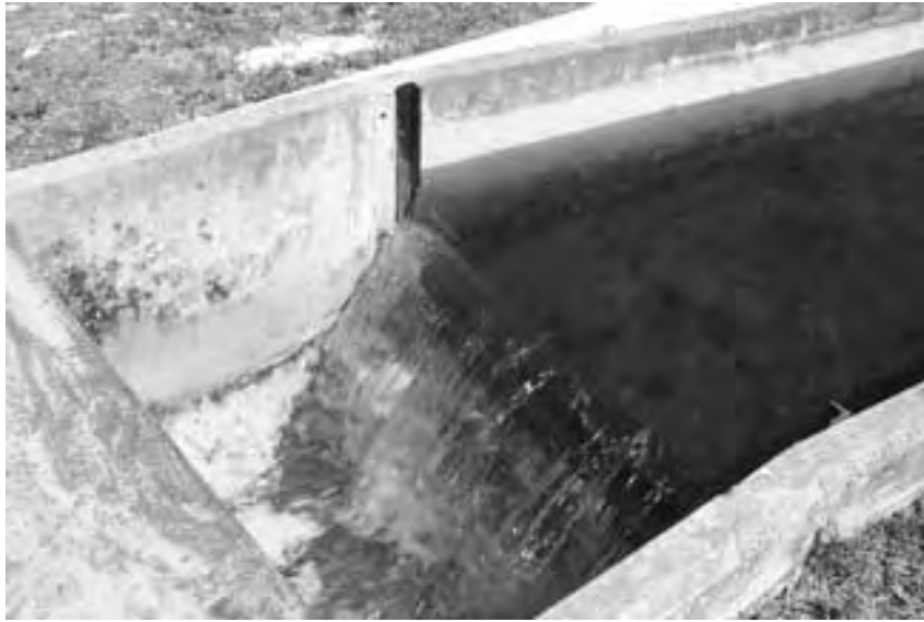
Figure 3.12: Thin-plate weir used for flow measurement
