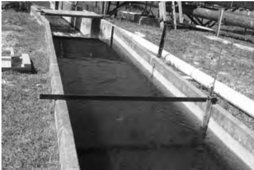
Figure 3.13: Water flowing in the direction of the weir. The point gage and stilling well are shown on the right of the picture
