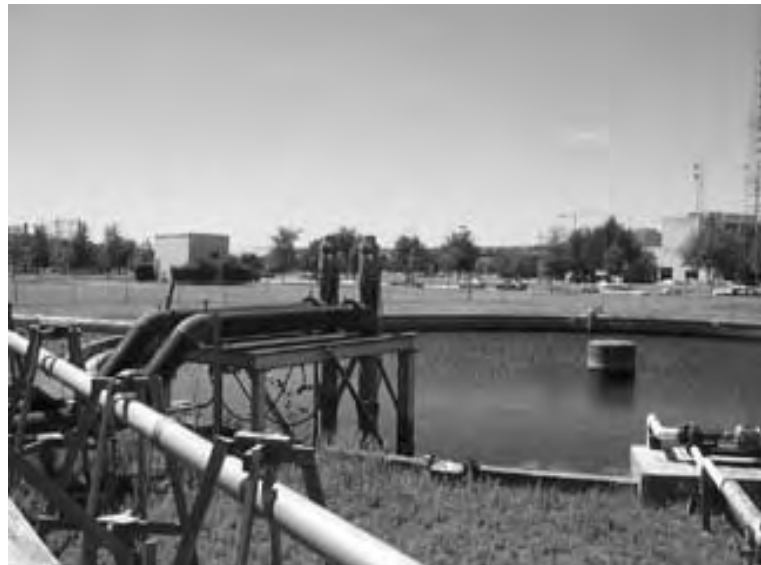
Figure 3.4: North (right) and South (left) pumps as installed on the reservoir
