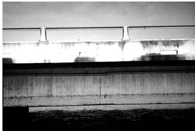
Figure 6.7: Disjointed conduit segments
