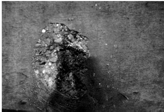
Figure 4.5: Typical spall in a footing
