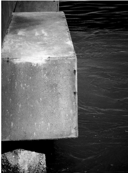
Figure 6.5: Corrosion of wire ties for Bent 21
