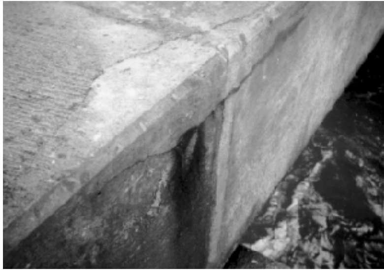
Figure 4.6: Crack in the proximity of tie beam construction joint
