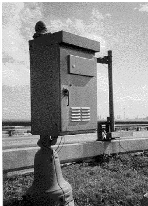
Photo 2.5 Outside of the Cabinet
