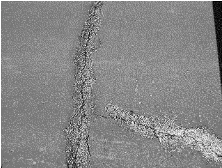
Figure 5.32. A Sealed Branched Crack
