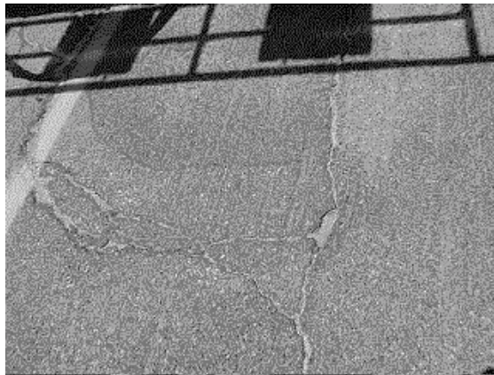
Figure 5.13. The Wide and Non-Uniform Cracks before Sealing
