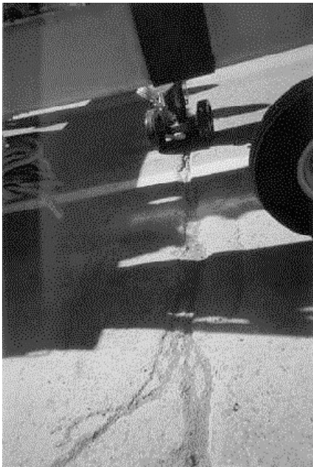
Figure 5.23. A Deep and Wide Crack before Sealing
