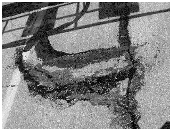
Figure 5.14. The Wide and Non-Uniform Cracks after Sealing
