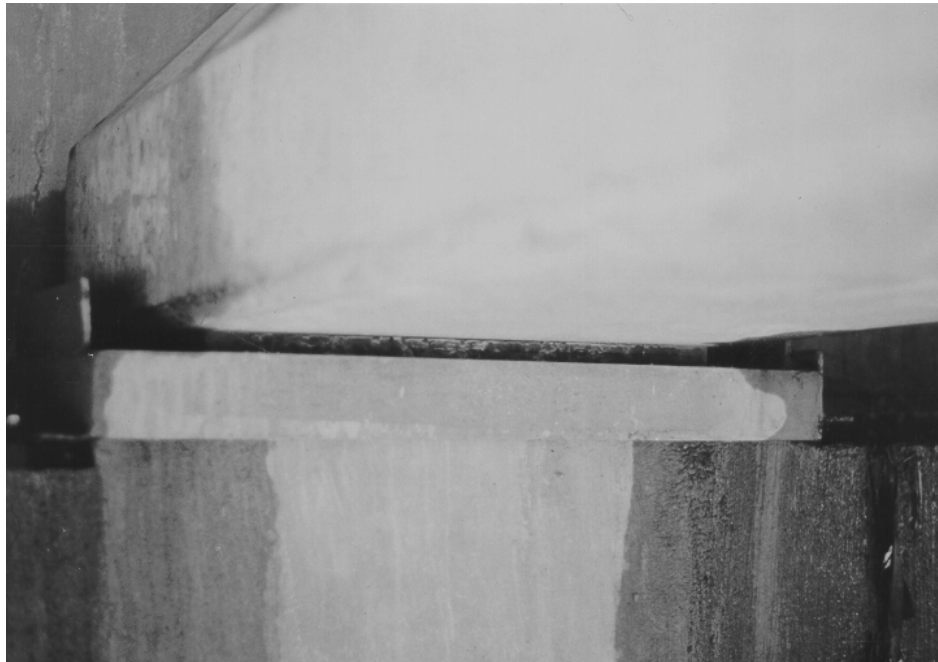
Figure 3- 11 Restraining devices to prevent bearing movement
