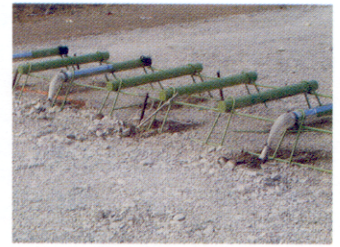
Figure 6—Instrumented Dowel Bars
