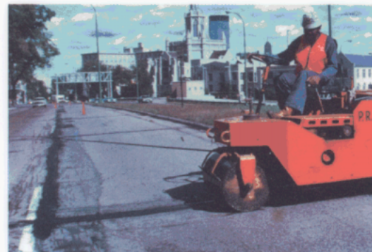
4 Compact the hot mix with roller so that patch is flush with adjacent pavement.
