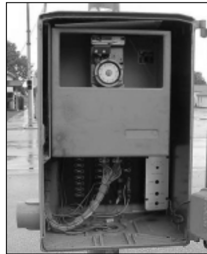
Figure 6 Controller Cabinet at Intersection 06
