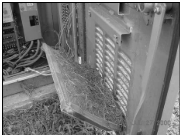
Figure 10 Dirty Filter at Intersection 14
