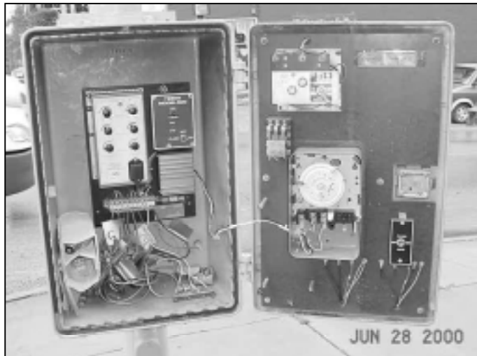
Figure 3 Controller Cabinet for Intersection 05
