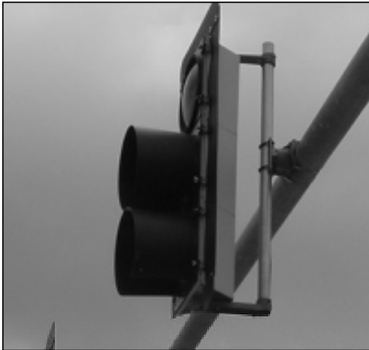
Figure 7 Missing Visor on Mast-arm Signal at Intersection 10
