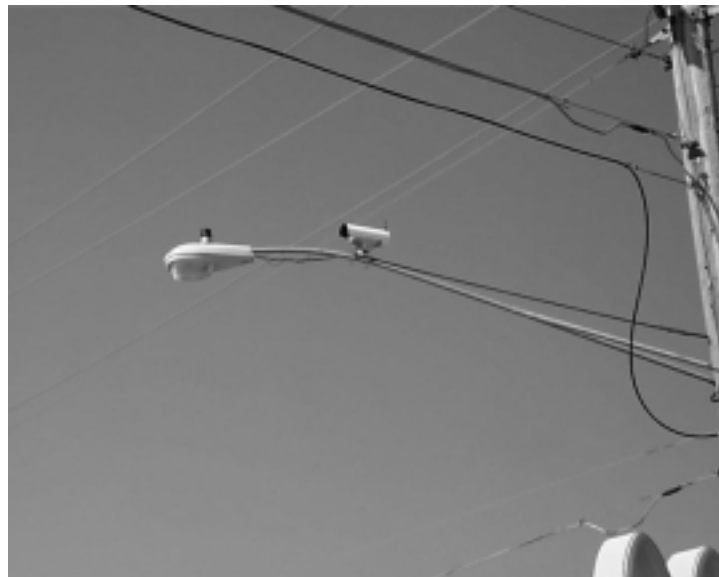
FIGURE 3.4 Camera placement on a street light mast arm.
