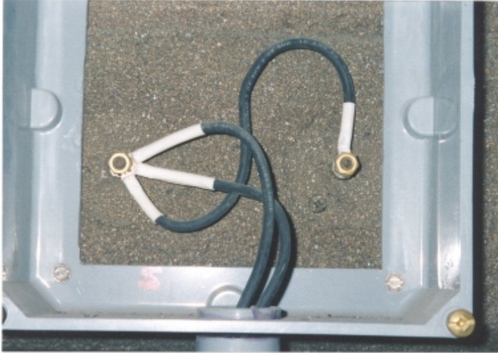
Figure 6.3: Flush-mounted current distribution plates with temporary wiring installed.
