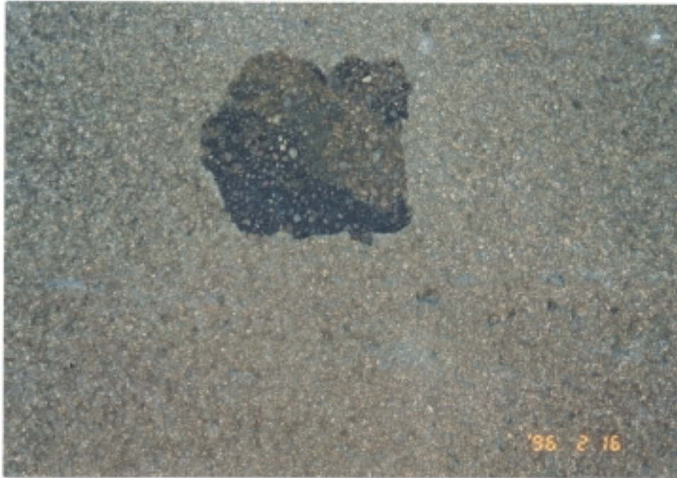
Figure 6.5: Typical disbonded area
