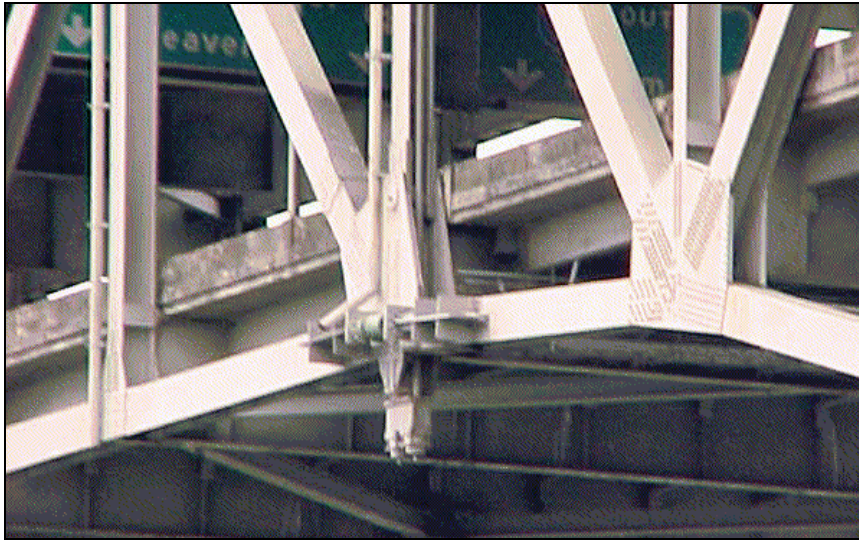
Figure 3.11: Shock Transmission Unit at Panel L13
