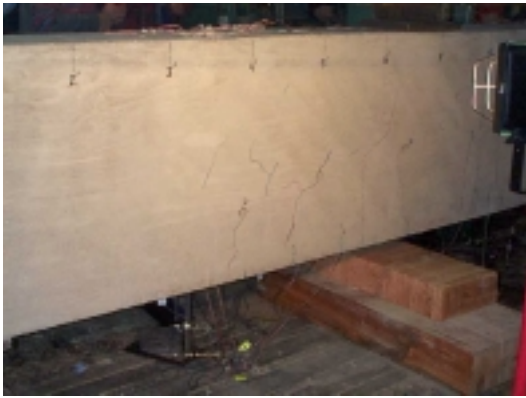
Figure A-20: Early cracking of Control beam
