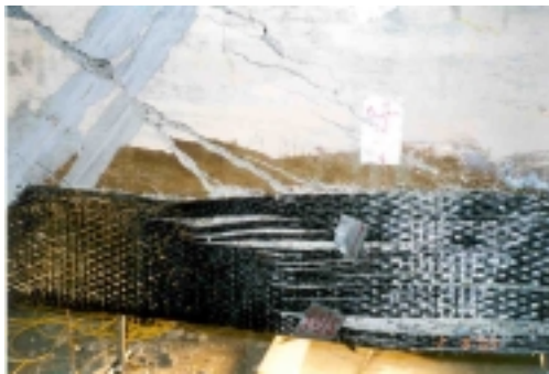
Figure A-32: CFRP transverse rupture
