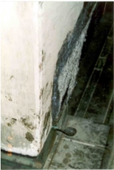
Figure A-37: Debonding of CFRP at support
