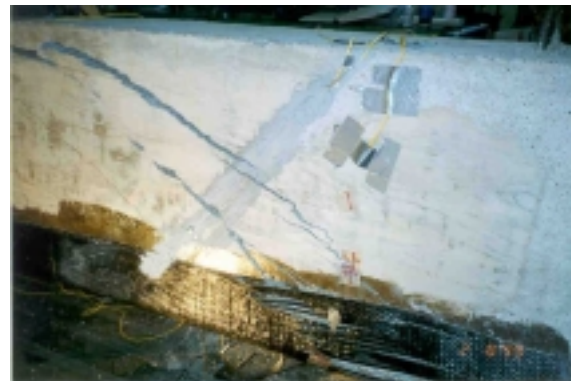
Figure A-30: Diagonal tension failure
