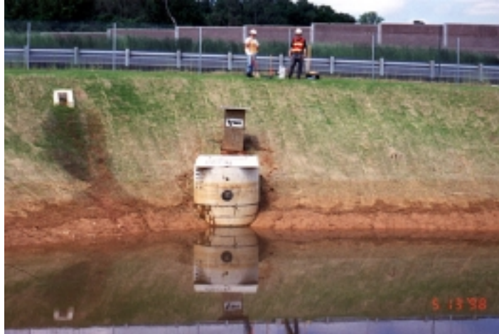
Figure 8. Outlet Riser Structure, Automatic Sampling Equipment Location, and Sampling Location
