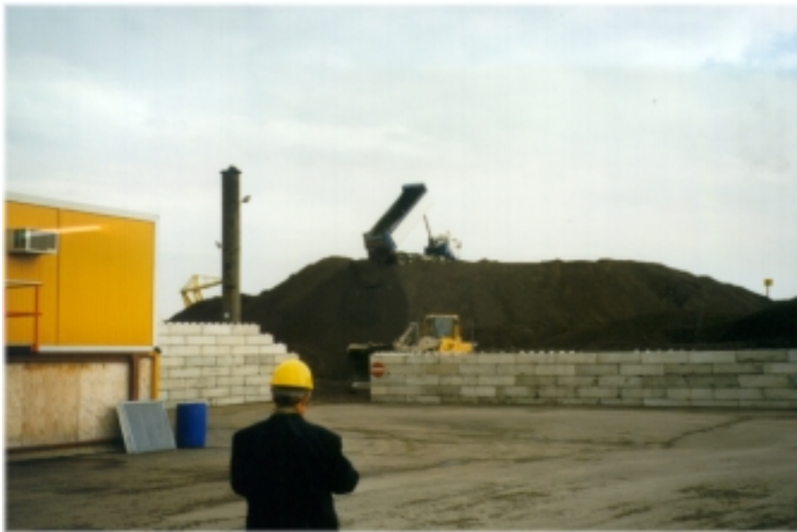
Figure 22. RAP is used at high substitution levels at the Swiss-designed Ammann double drum hot recycling asphalt plant in the Netherlands.
