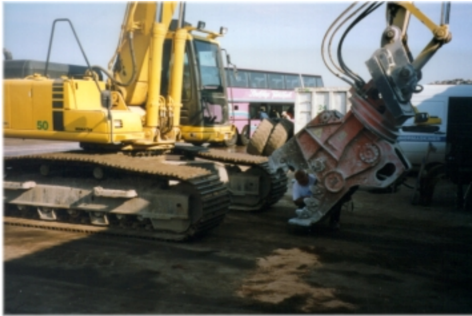
Figure 11. Concrete jaw crusher at the RGS 90 A/S materials processing plant in Denmark.
