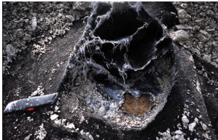
Figure 28. Top-membrane tear, caused by a bucket loader.
