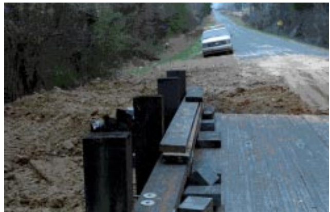
Figure 9—Attachment of bridge curb and rail system following the second bar tensioning.
