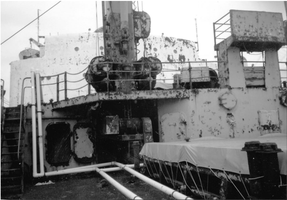
Figure 3: Deteriorating Vessel at MARAD's James River Reserve Fleet
