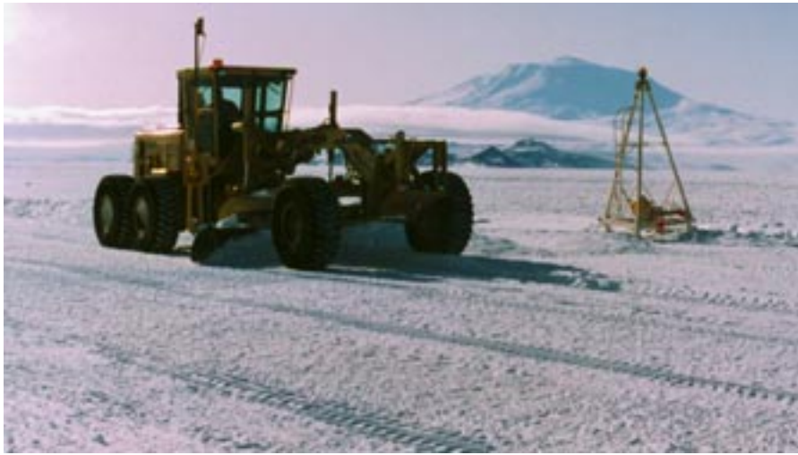
Figure 44. Motor grader under laser control during final grading of ice. Transmitter is mounted on robust, portable tower.
