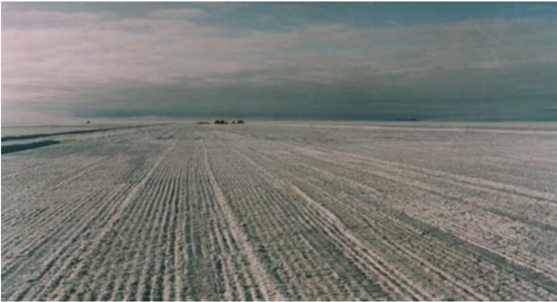
Figure 47. Finish-graded ice surface seen in foreground with rough graded segment of runway in background.
