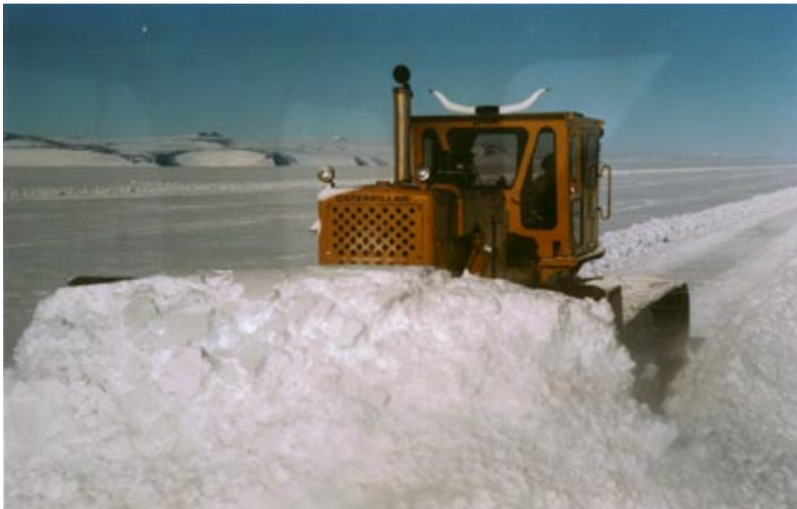
Figure 28. Initial snow stripping on the Pegasus runway using a bulldozer with U-blade.
