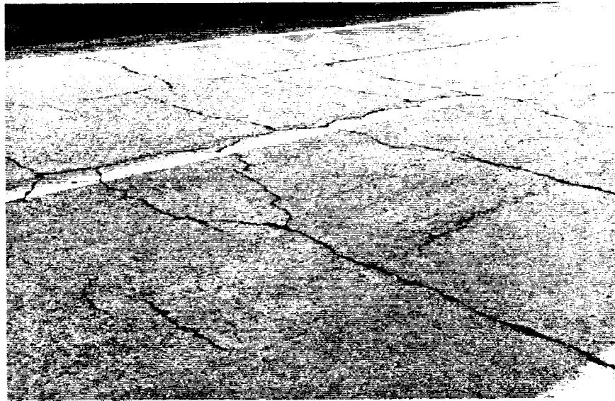
FIGURE 2. Asphalt T-1 in both lanes showing transverse cracking
