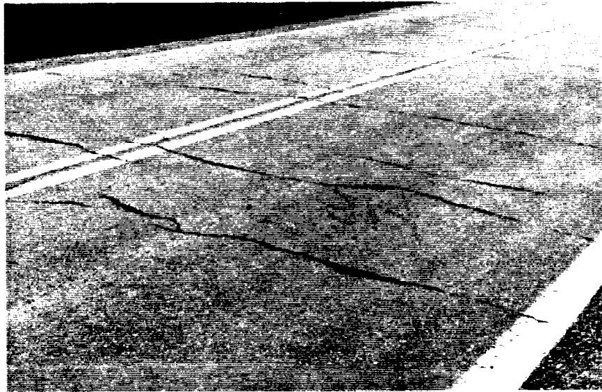
FIGURE 4. Asphalt T-5 in both lanes showing well-defined full- and half-width transverse cracks.
