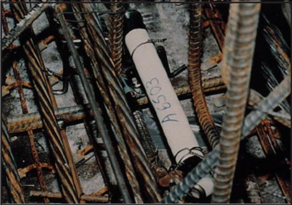
Figure 2. Carlson Strain Meter. The gage is located in the bottom flange of a prestressed concrete girder.
