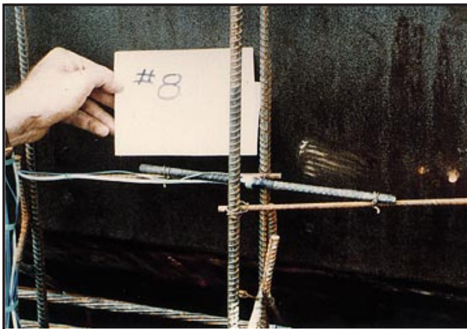
Figure 4. Electrical resistance strain gage and Carlson Strain Meter. Both gages are located in the deck slab above a prestressed concrete girder.
