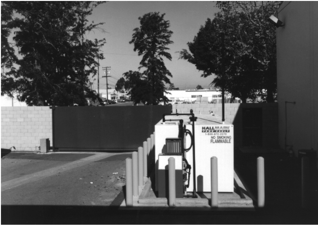
Figure 14. An above-ground tank and dispenser were installed for the M-85 fueling facility.
