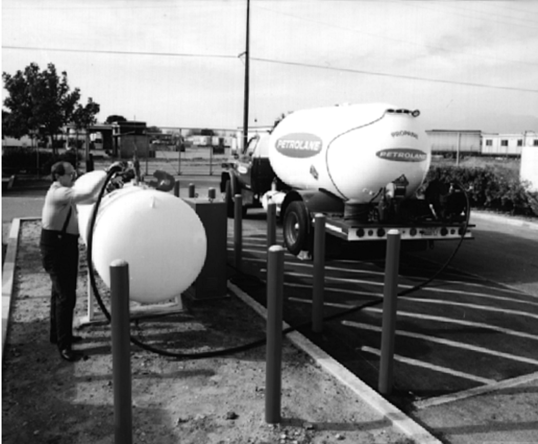
Figure 13. The propane gas fueling facility was located on an island in the parking lot.
