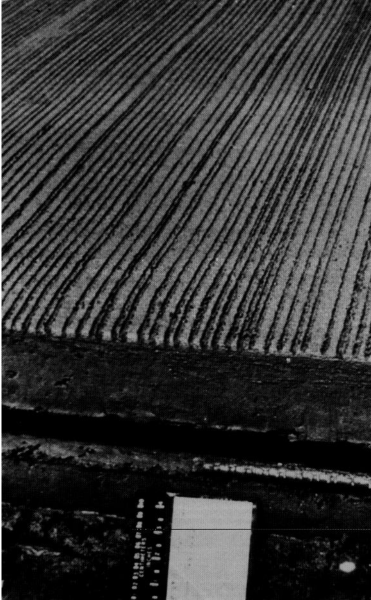
FIGURE 2-5. WIRE COMB TECHNIQUE CONSTRUCTED AT PATRICK HENRY AIRPORT, VIRGINIA, USING A 1/8 INCH X 1/8 INCH X 1/2 INCH CONFIGURATION
