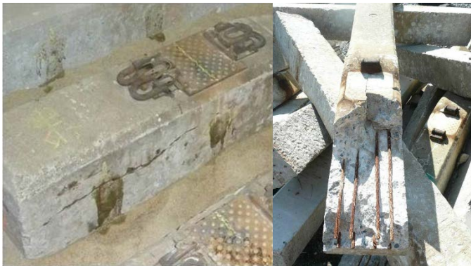
Figure 1: Horizontal splitting cracks in concrete crossties on Amtrak’s Northeast Corridor [3].
