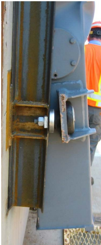
Figure 8. Post-test Photograph Showing Tank Pulling Away from Wall
