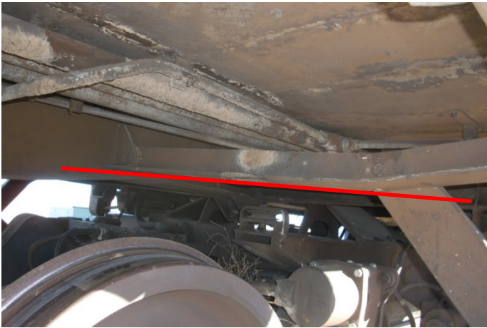
Figure 14. M1 underframe member bent near front truck connection, left side
