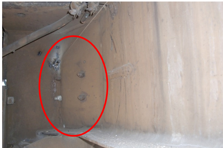
Figure 7. Bulging of M1 left draft sill due to coupler shank pushing on coupler stops inside bellmouth
