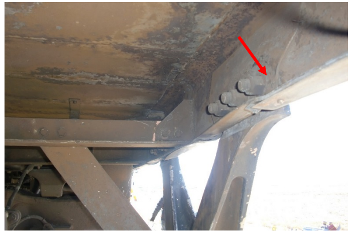
Figure 12. M1 side sill buckled at front left truck connection (interior view)
