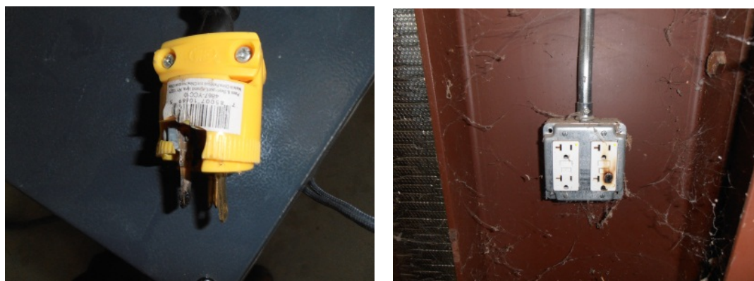
Figure 3: Burned plug and outlet at Sacramento NWR
