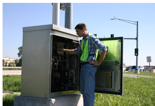
Figure 19 Operation Green Light technician adjusts signal timing at traffic signal cabinet. Source: MARC
