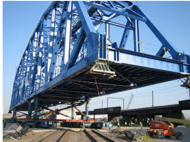
Figure 14. CREATE grade separation project GS15a under construction at 130 th St. and Torrence Ave. in Chicago. Source: CREATE
