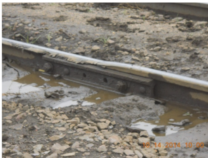
Figure 1: Mismatched Joint with Ramp
