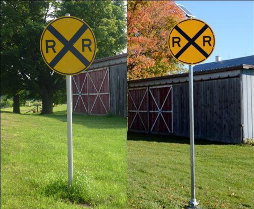
Figure 9. Lakewood Drive Northbound Approach Advance Warning Sign Before (Left) and After (Right) LED Sign Installation
