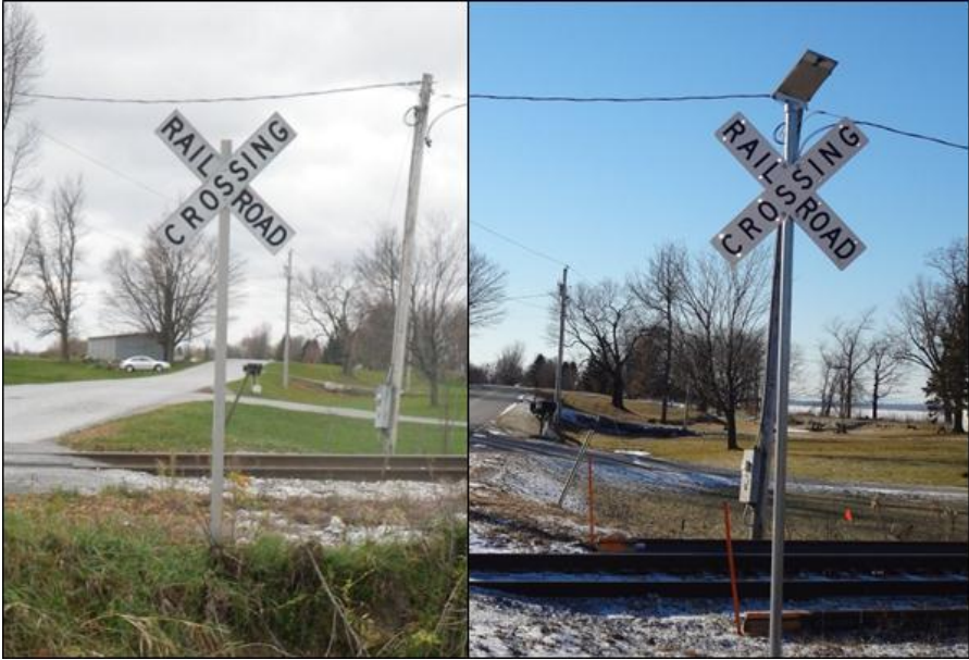
Figure 8. Lakewood Drive Southbound Approach Crossbuck Sign Before (Left) and After (Right) LED Sign Installation
