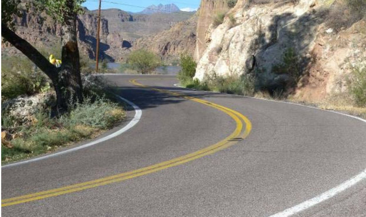
Figure 7: One of the paved hazardous curves identified in the RSA (Location #8, Source: RSA).
