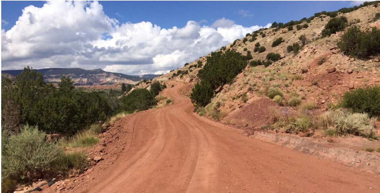
Figure 3: FR 151 Conditions at Mile Post 6, one of the steepest sections of the road.
