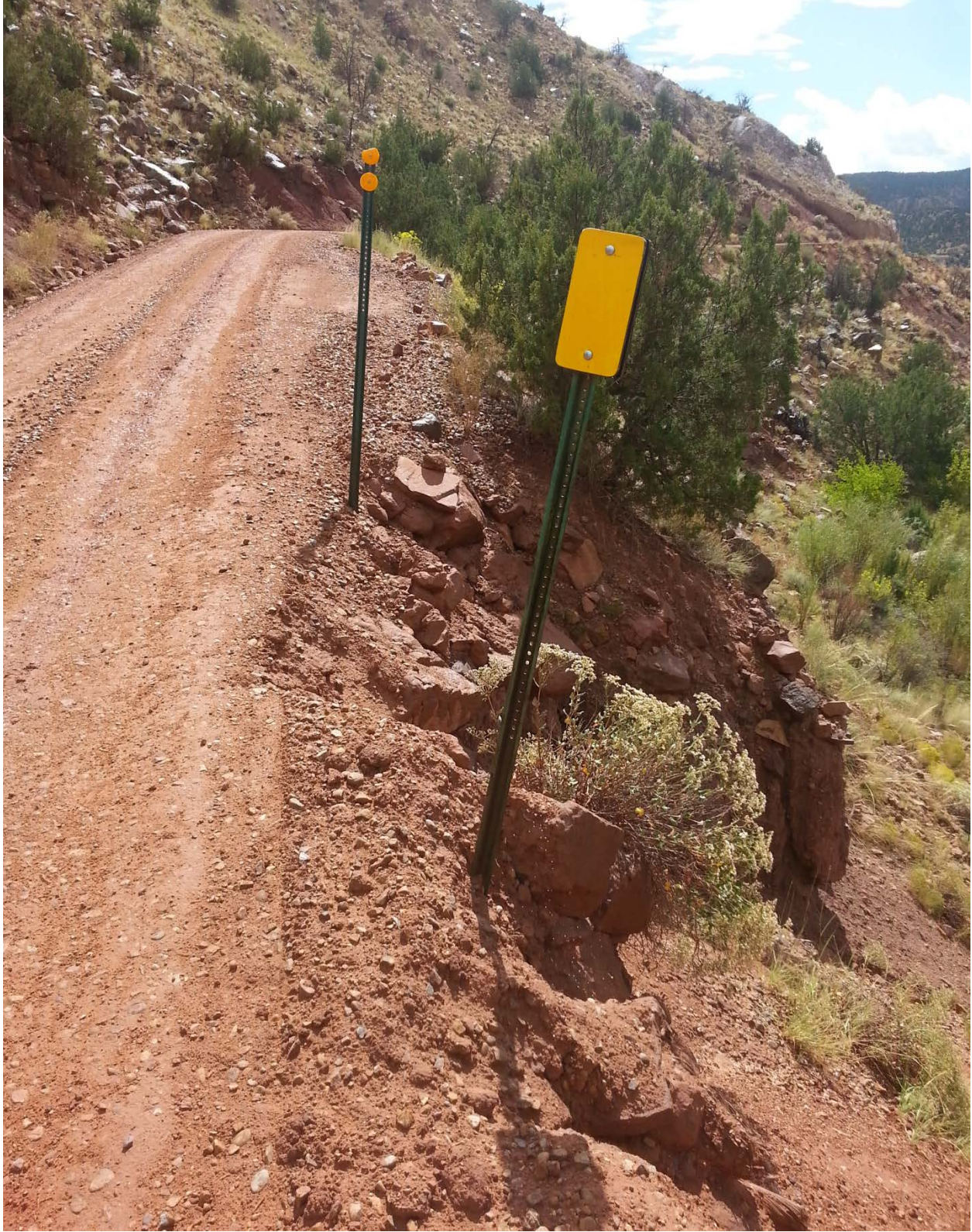
Figure 8: Existing delineators along the edge of eroding roadbed near Mile Post 6
