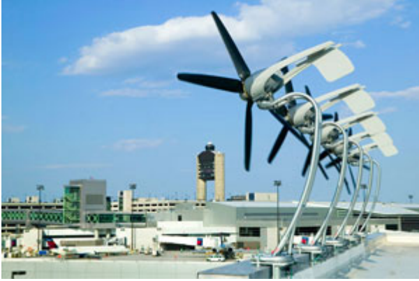
Figure 24. Small, Residential-Scale Wind Turbines at Boston Logan International Airport
