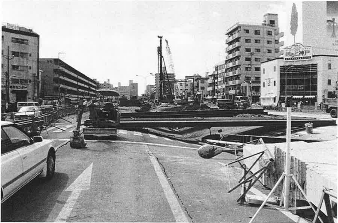
KMS-1. Depression in the street is above the Daikai-dori Station.
