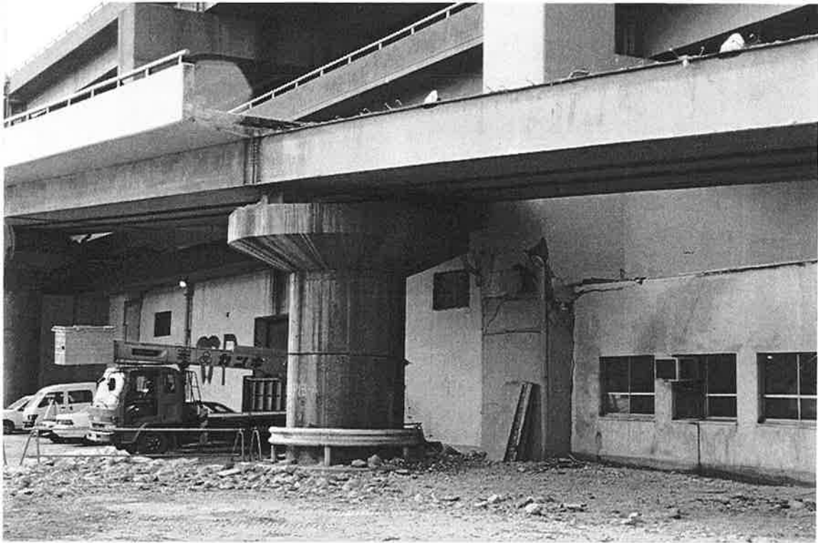
PI-17. This highway ramp adjacent to the peplemover appears to be supported on a seismic isolation bearing. The deck was damaged here and demolished. The concrete substructure of the double viaduct sustained significant damage.
