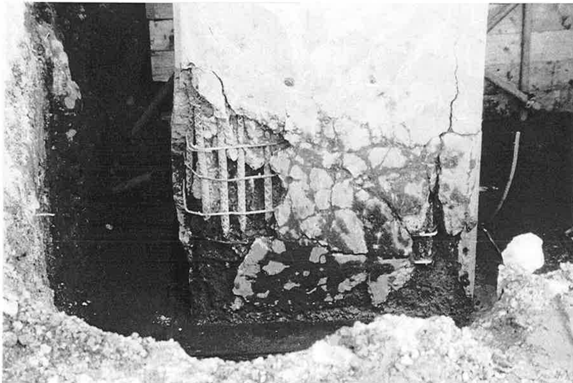
JRS-18. Some spalling is evident at the bottom of this column. Note the tie size and spacing.
