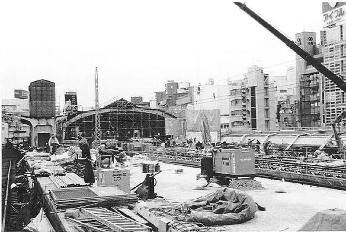
SS-3. The ballast and trackwork has been replaced on the turnouts leading into the maintenance facility. The supporting girders fell to the street.
