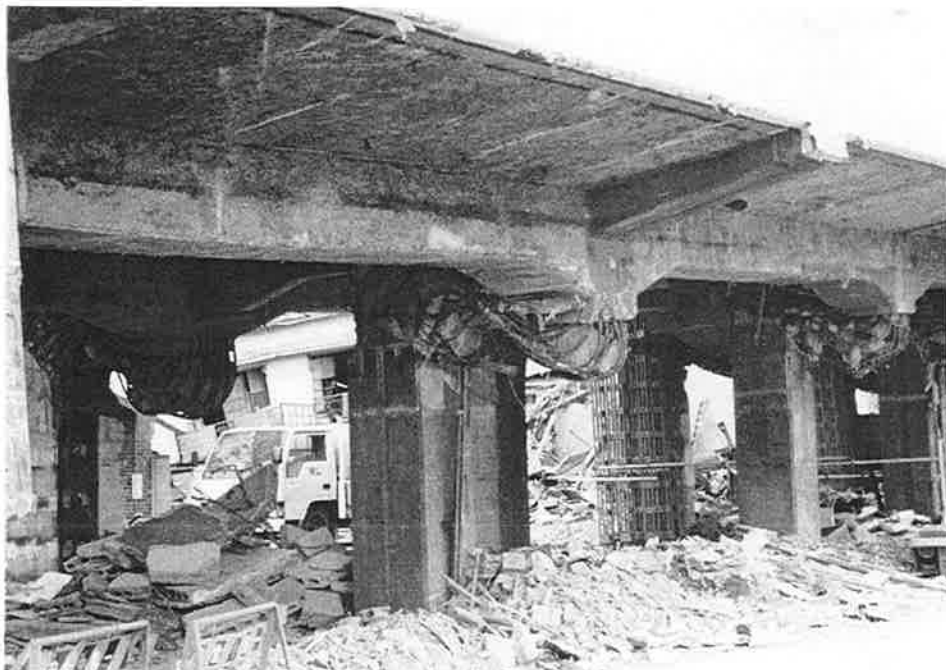
HER-26. Another failed viaduct section; some of the debris is consistent with the additional use of the facility.
