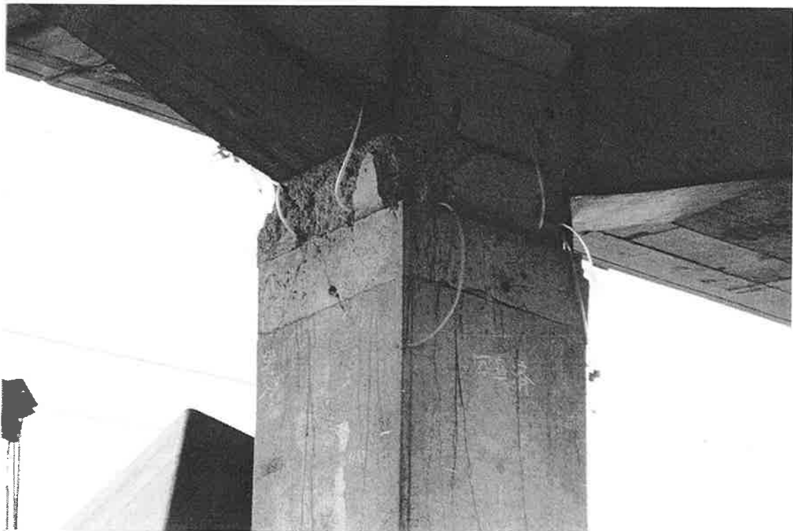
JRS-30. A close up photo of minor longitudinal damage on the column
