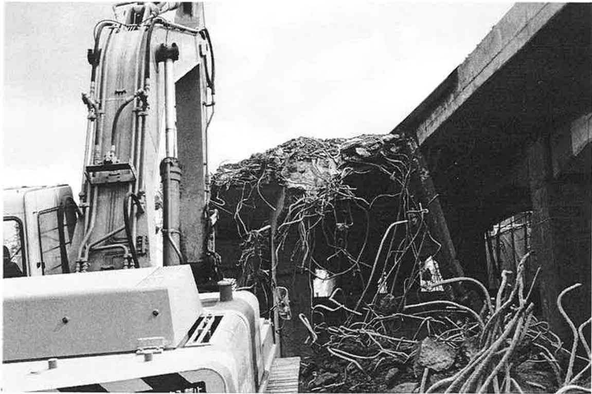
HC-8. Demolition of the final section of concrete viaduct. Note the clean edge separating the parallel structures.
