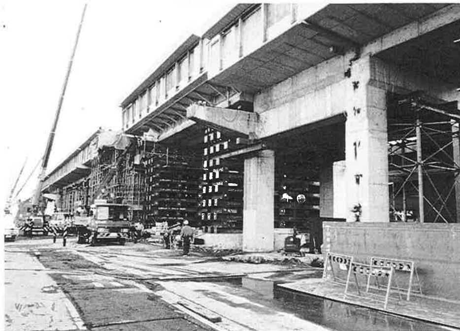
JRS-16. The drop-in span has been lifted from the ground while the superstructure is finished.
