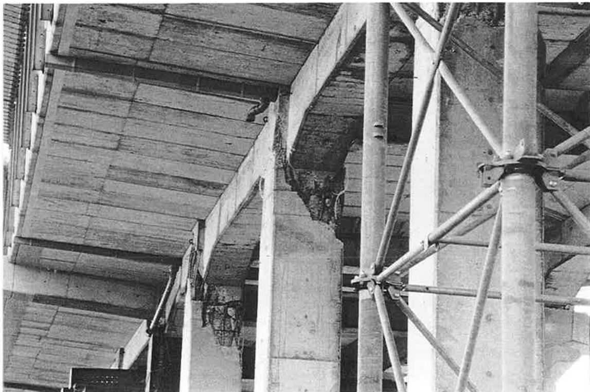
JRS-4. These columns show primarily transverse damage, but also some horizontal spalling.
