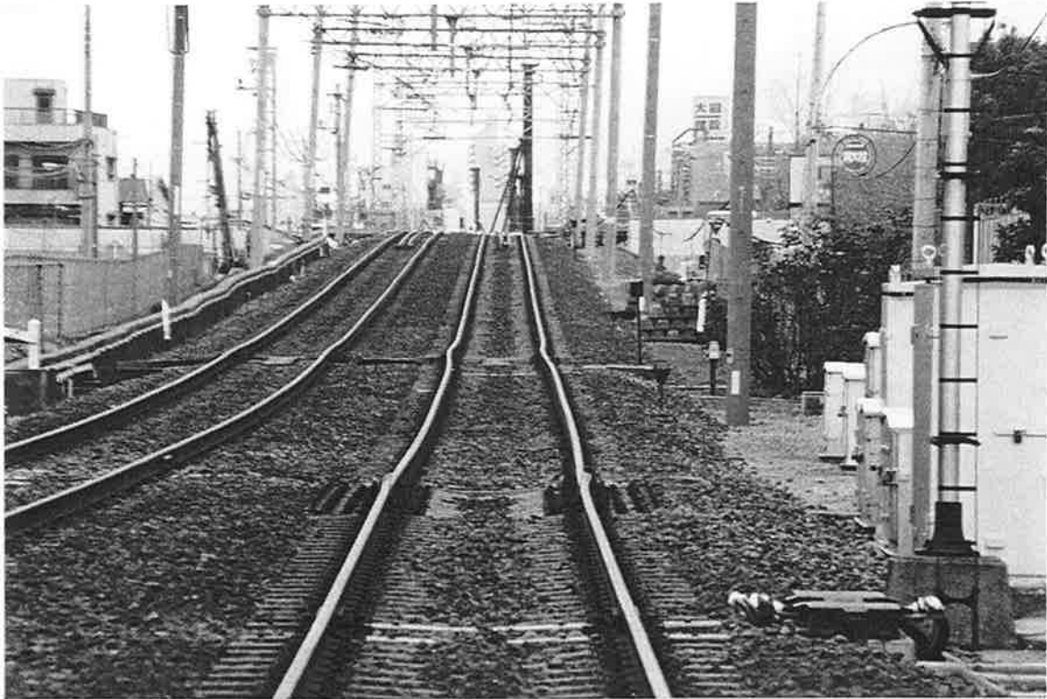
HC-4. Displacement in rail near Nishinomiya Station
