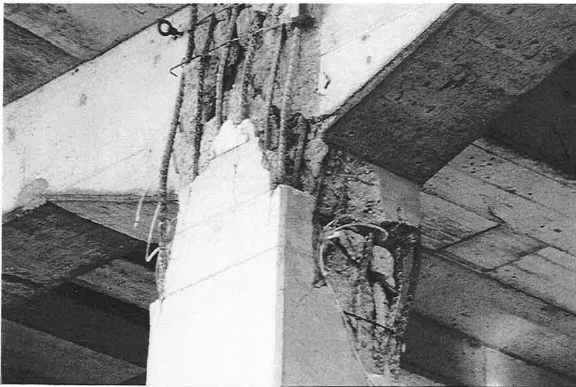
JRS-5. Column very close to collapse with diagonal cracks through the joint zone and ties ruptured; the joint is badly deteriorated.
