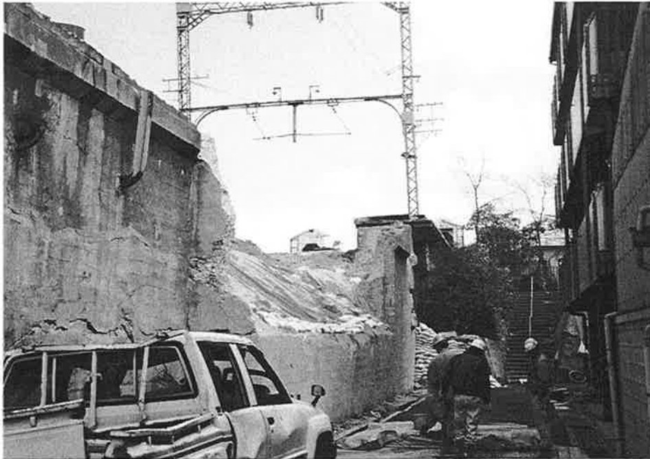
HER-5. Another section of failed gravity retaining wall; there is another failed section above the sandbags in the background. Note the horizontal crack above the parked vehicle.
