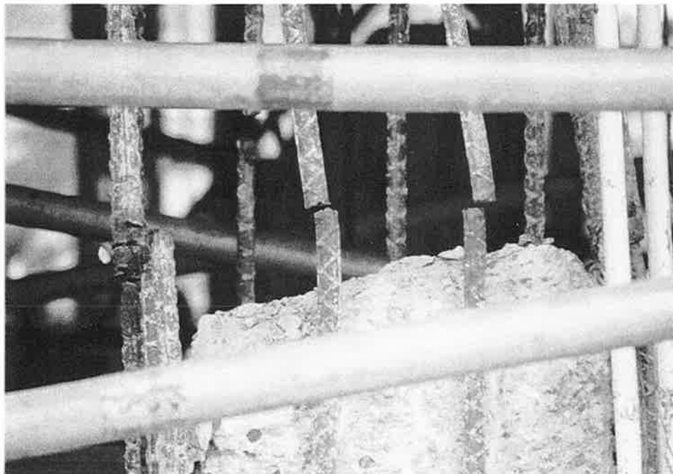
JRT-26. The center two column bars (transverse) appear ruptured while the left side (longitudinal) bars appear to have been flame cut.
