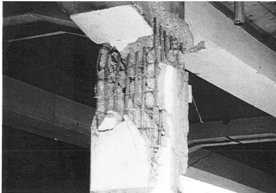
HER-32. Damage to a column west of Shinzaike Station; major transverse shear cracking and longitudinal spalling are evident.
