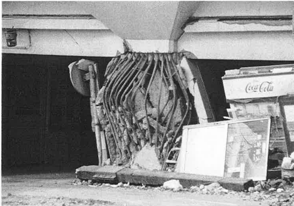
HER-13. Close up of the center column of the pier; the concrete wasn't properly confined and the untied reinforcing buckled.
