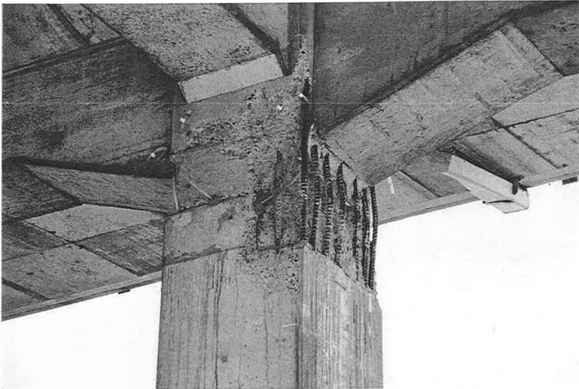
JRS-13. Column damage in the longitudinal direction
