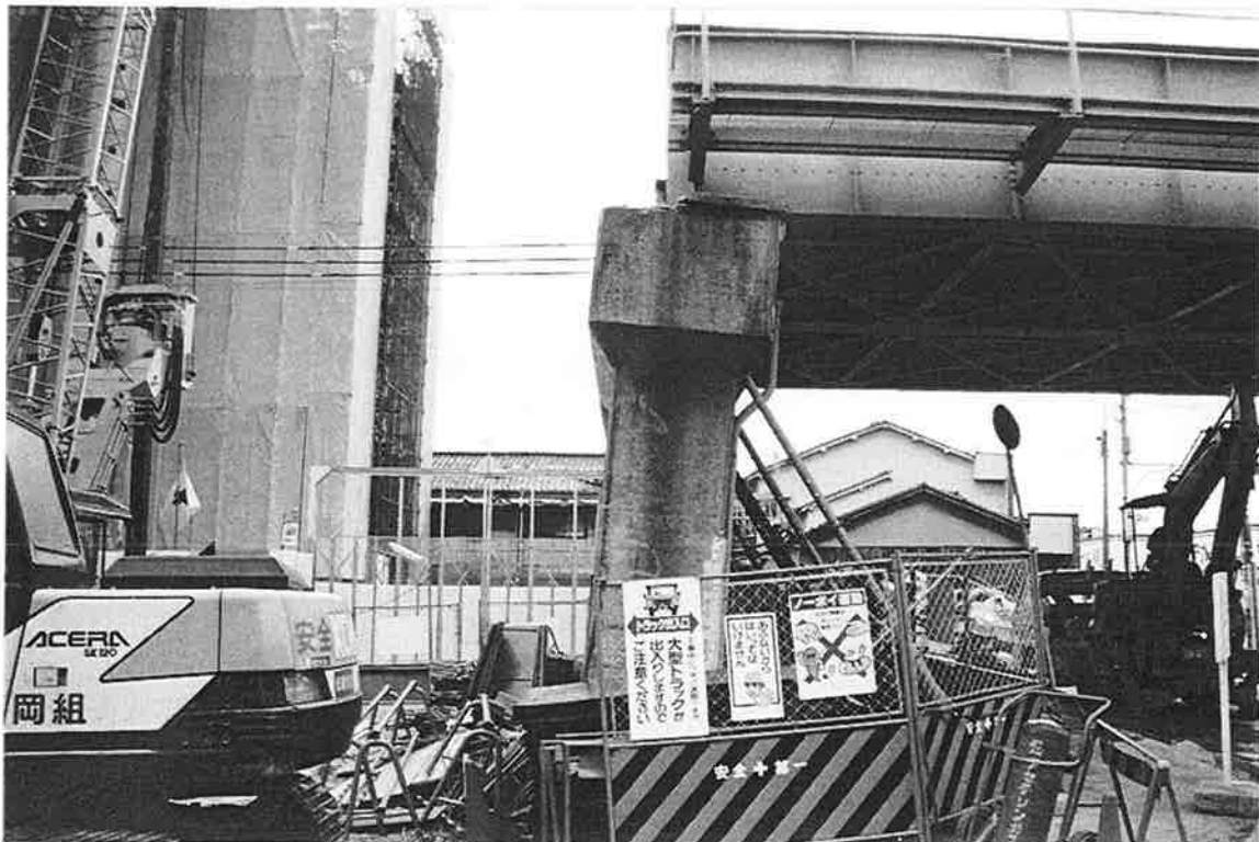
HC-9. The pier wall supporting this steel through girder is leaning significantly only at this end indicating the bearings slipped. The adjoining concrete structure was removed entirely.
