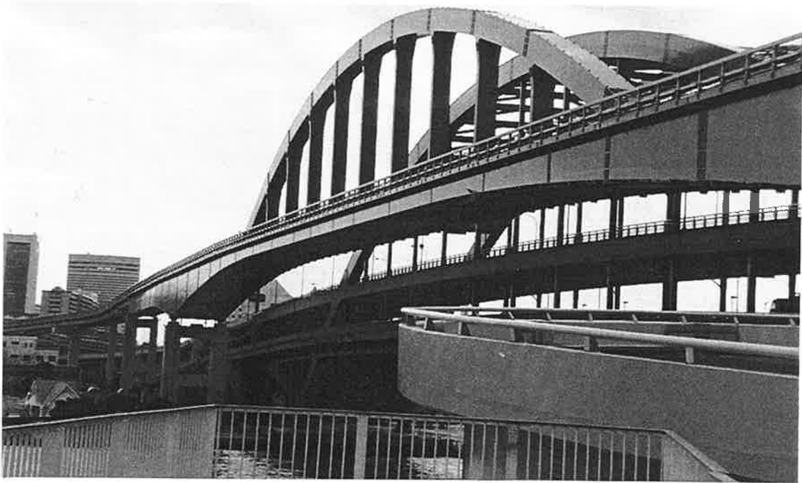
PI-13. The single arch bridge in the foreground carried the people mover south to Port Island. It appeared undamaged. The highway bridge at the bottom right was severely damaged in the next span. The double deck arch in the background supports highway traffic.
