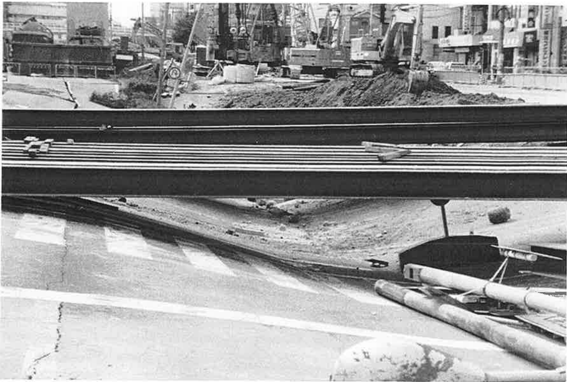
KMS-2. The steel sections over the depression are being used as soldier piles.
