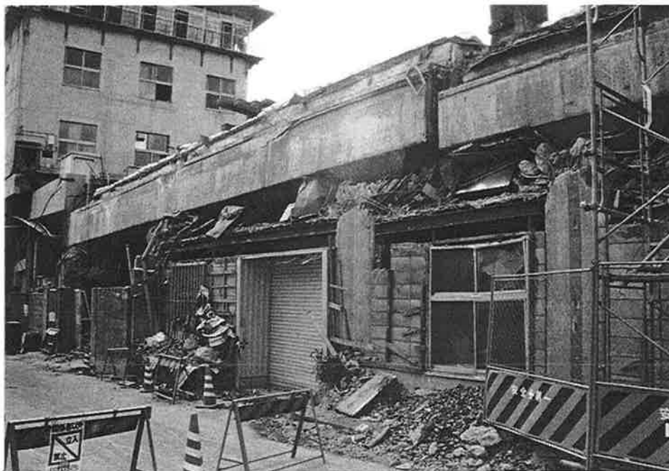
HER-16. This section is completely destroyed above the steel beams. The steel beams were installed for secondary uses of this facility. The beams seem to have concentrated the damage at the tops of the columns. This section was some sort of siding ending at the building.
