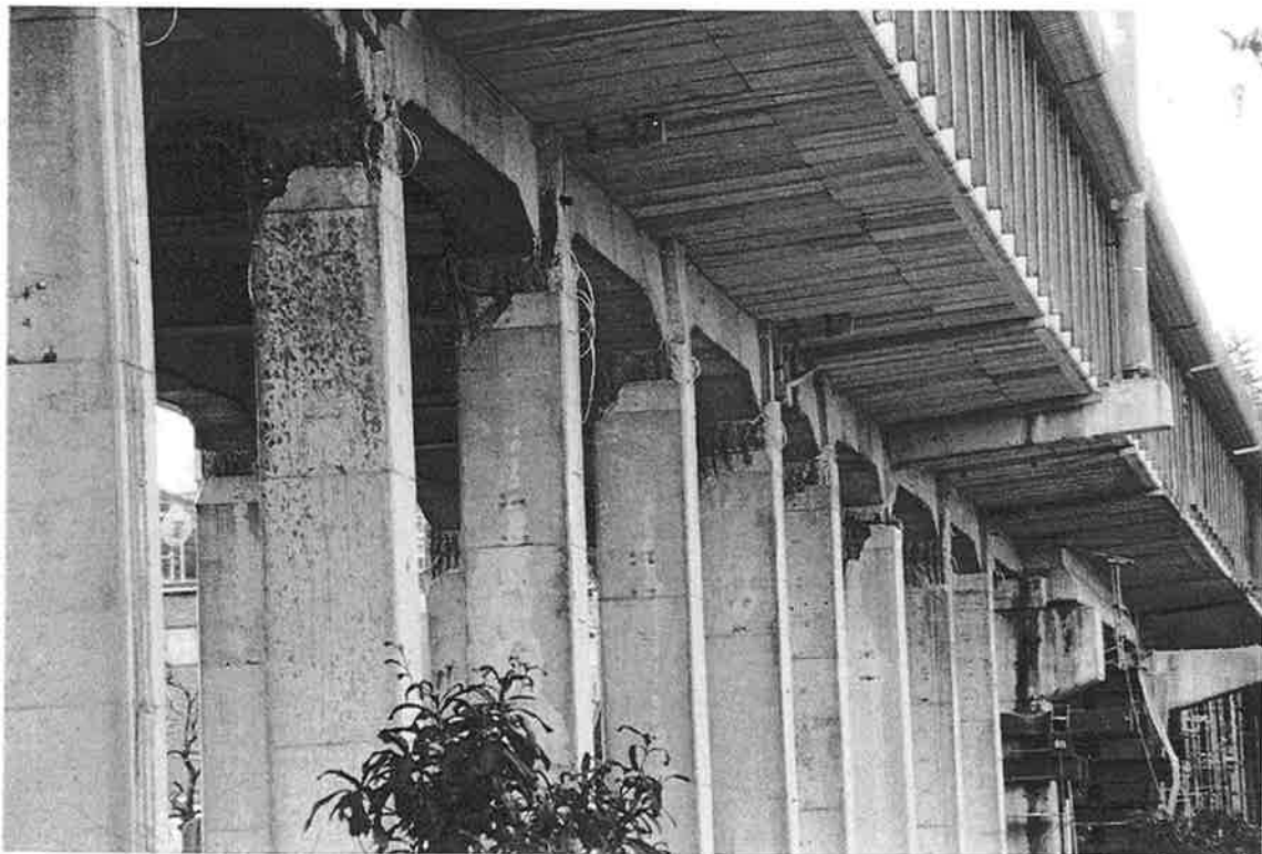
JRS-28. Longitudinal response is shown by the damage in consecutive columns. There is minimal transverse damage.
