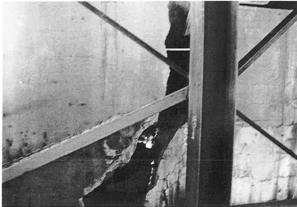
HER-4. This 150 mm wide crack is in an abutment wall at the west end of the failed retained embankment. The steel column is supporting the superstructure of the street crossing.
