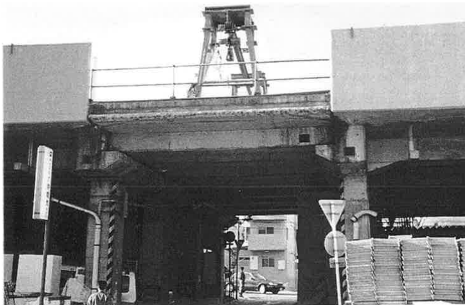
JRT-42. This drop-in span was lifted back into position. Note the seat lengths.
