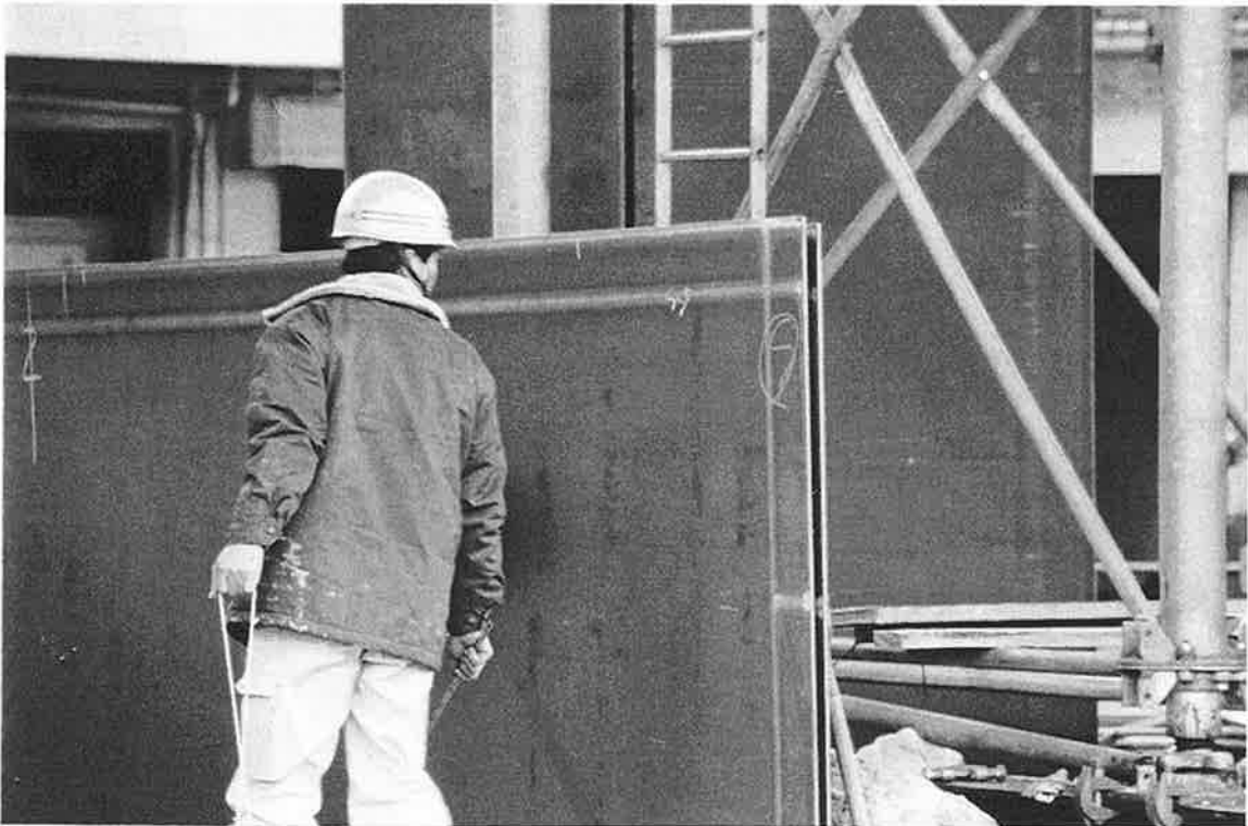
JRS-17. This construction worker is standing on a steel jacket. The jacket is nearly 1.5 meters on a side and only 9 mm thick.
