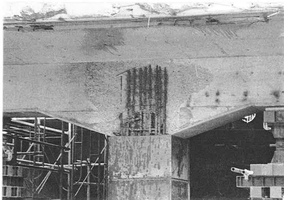
JRT-24. The square steel plate jacket extends to the top of column. The column bars are exposed through the joint to the termination.
