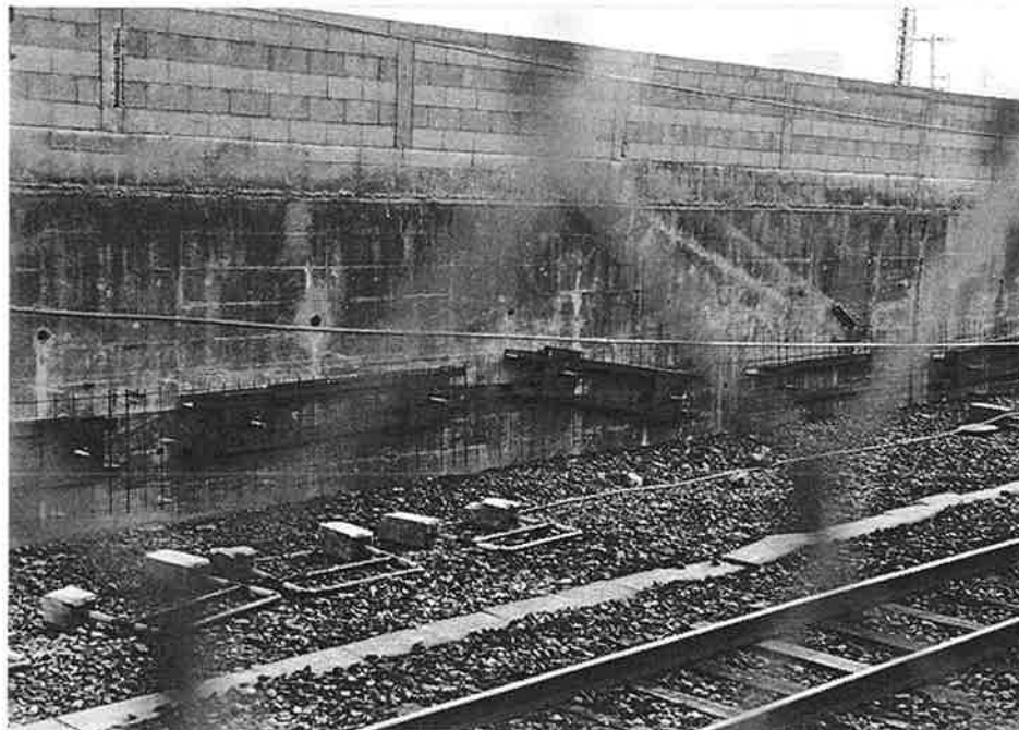
JRT-4. Retaining embankment through bolts as seen from the back face of the wall.
