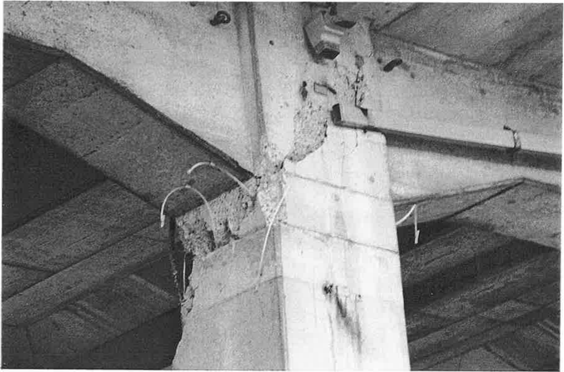
JRS-25. The cracks have been epoxy grouted. The external spalling still needs repair.
