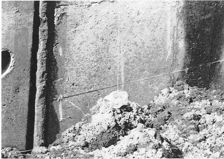
JRT-3. This concrete plumb bob indicates a 400mm lean in the retaining wall.
