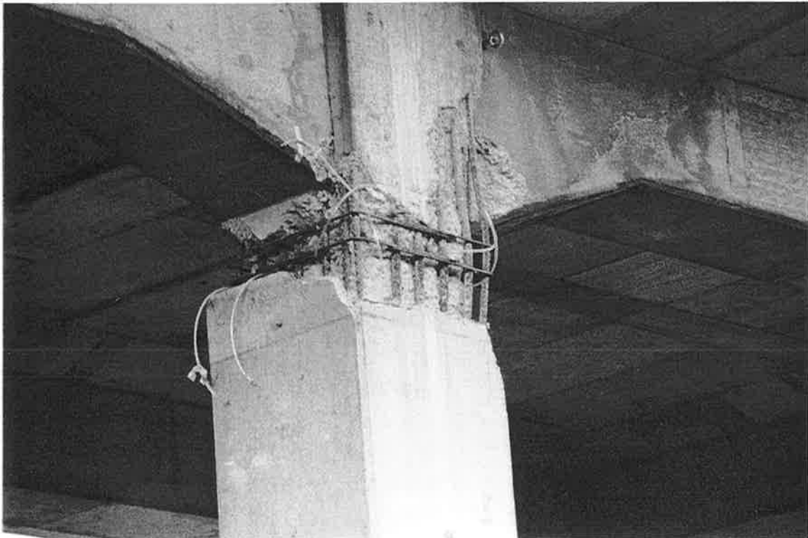
JRS-2. Another column damaged and grouted
