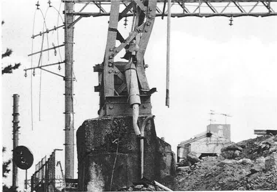
HER-7. The column of the catenary support observed earlier has buckled.
