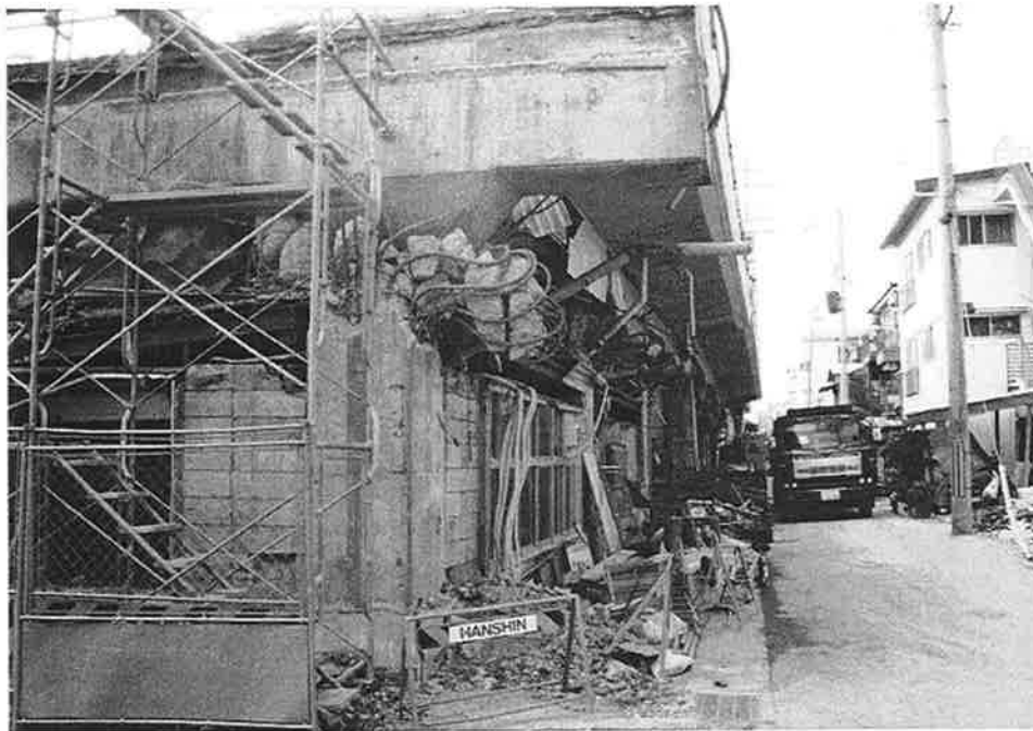
HER-17. Another section that collapsed above the steel beams; the fore span was a steel girder street crossing that fell and was removed. The truck at the right is being used to clear rubble so construction equipment can gain access.
