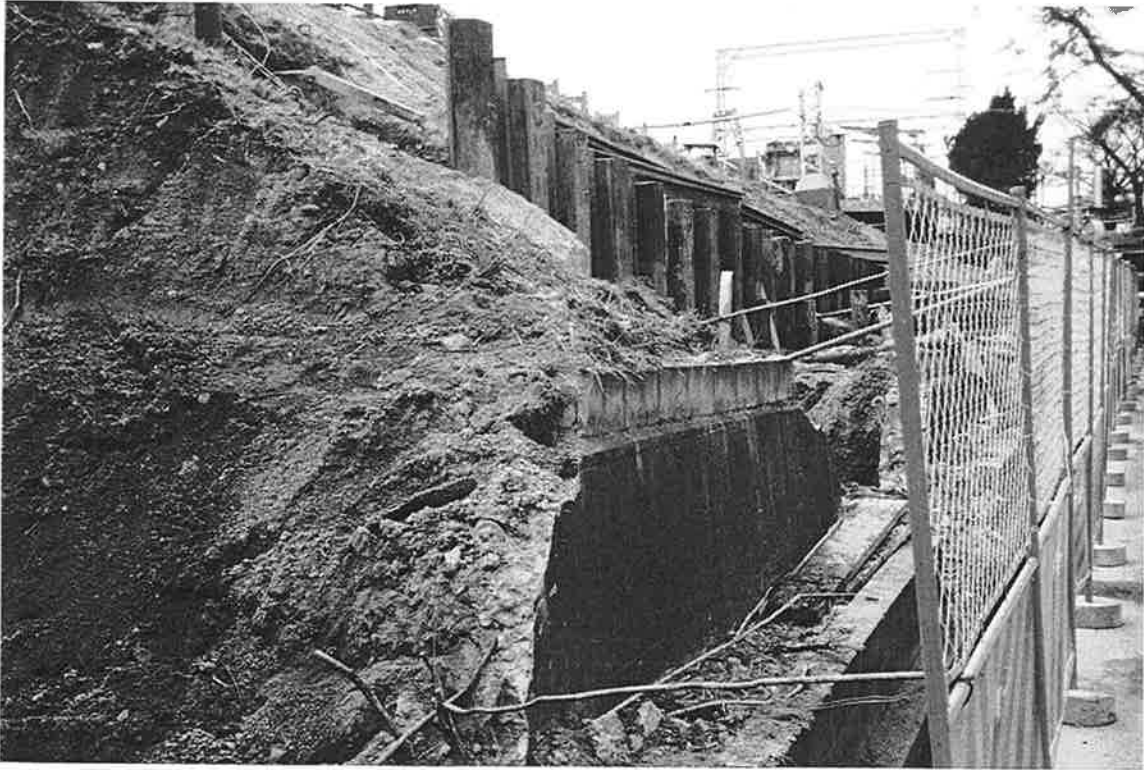
HC-10. Failed retaining walls near Shukugawa Station
