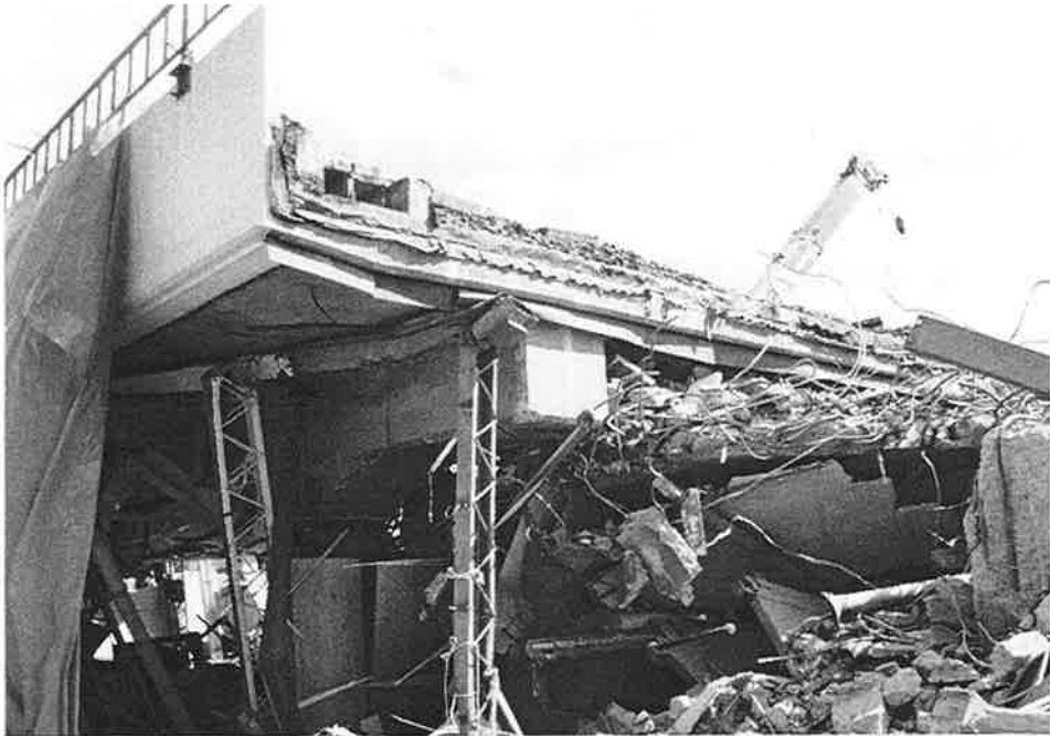
HER-11. The viaduct collapsed to the left of the expansion joint but was destroyed to the right. The joints were located at midspan. The ballasted rail provided no restraint.
