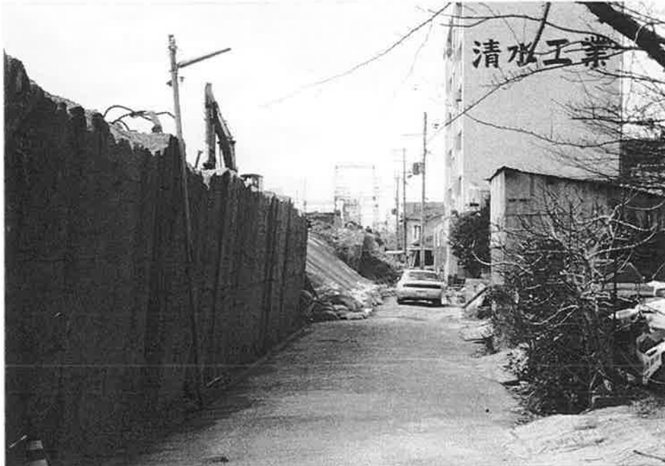
HER-8. Another retaining wall failure
