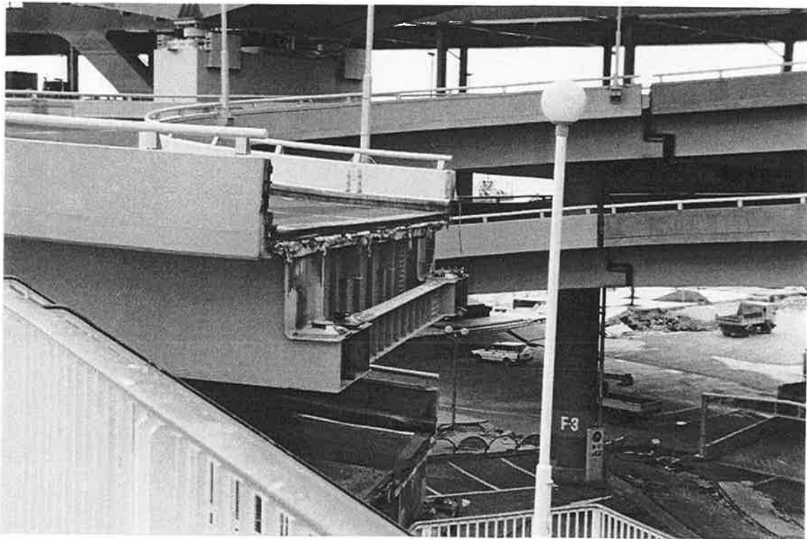
PI-14. These spans of the double deck highway bridge fell from the short span bridge seats. The arch bridge pier is at the top.
