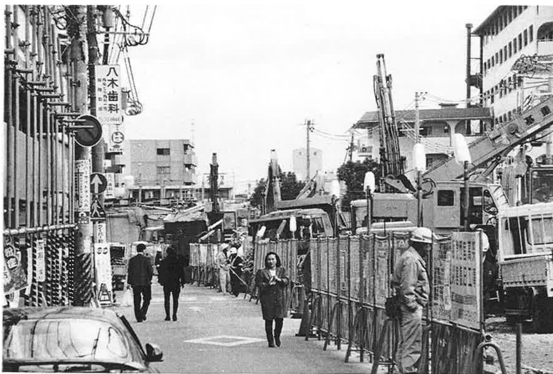
HC-14. This very crowded new construction to replace the demolished viaduct is between minimally damaged residential and light commercial use buildings.
