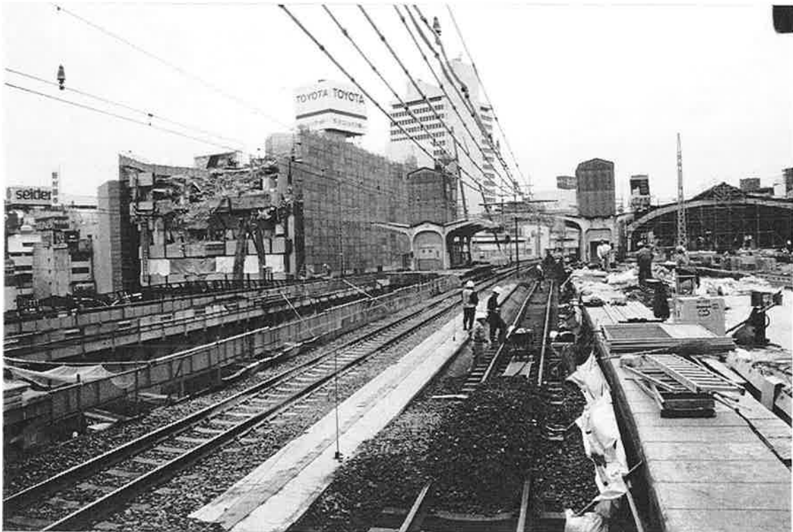
SS-2. The ballast is being replaced and recompact on the westbound track. Note the damage to the building to the left.
