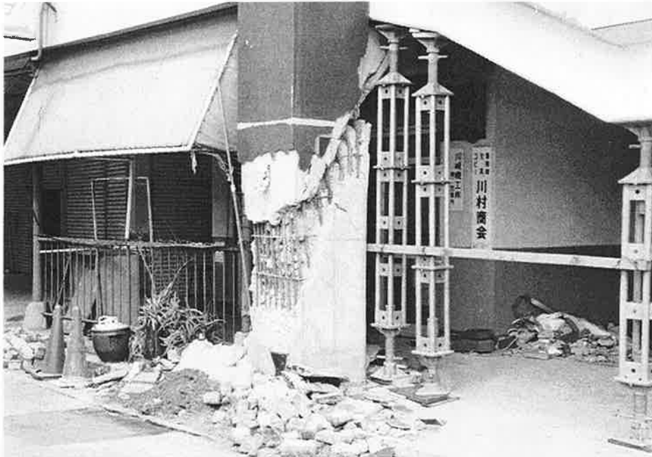
HER-29. A severely damaged column near Shinzaike Station entrance.
