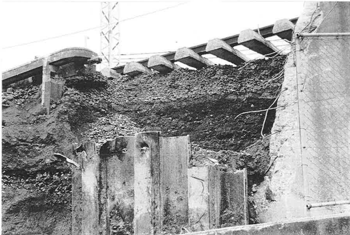
HC-5. Embankment failure undercutting concrete ties at an abutment near Nishinomiya Station
