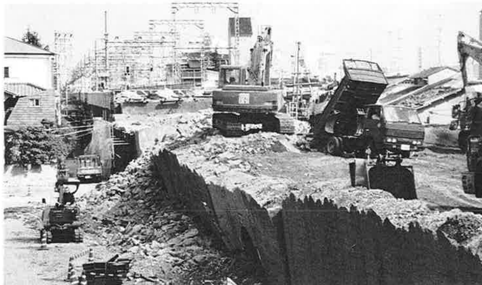
HER-2. More failed retaining walls; the embankment is being lowered to allow replacement of the walls.
