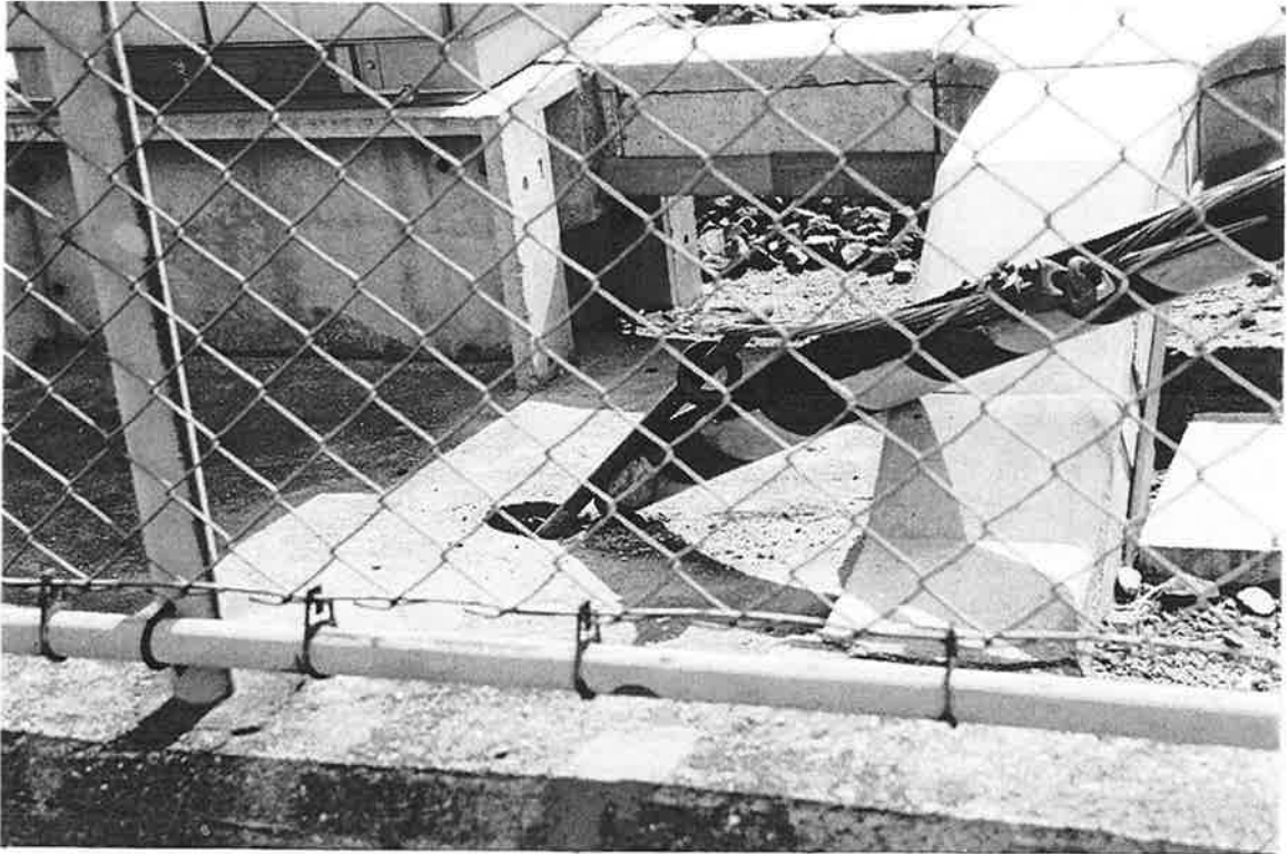
HC-6. Anchors pulled out of this electrification support stay allow the support tower to sway freely.
