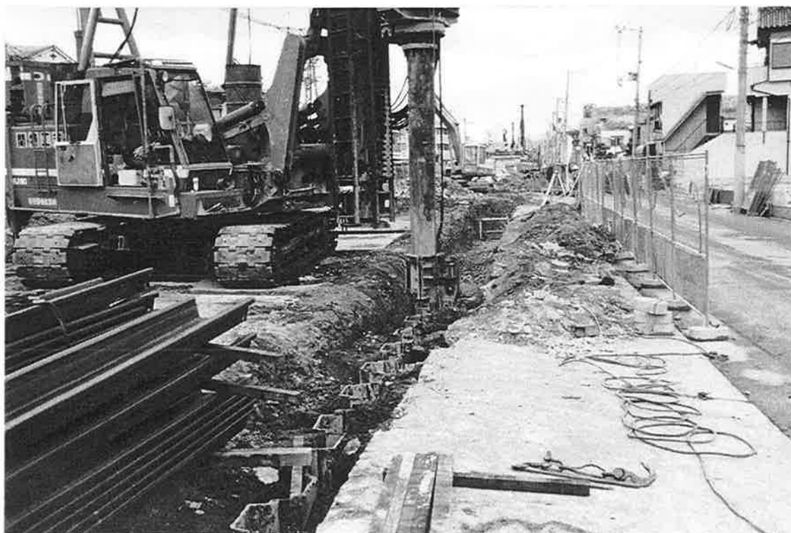
HC-15. New sheet piles being driven on the north side of the demolished viaduct.
