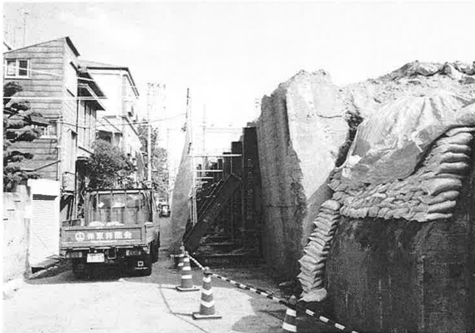
HER-1. Retaining wall west of Mikage Station; the steel frames resist additional leaning.
