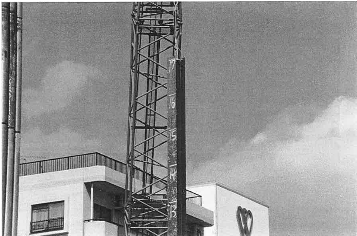
KMS-6. The new soldier piles are driven to 17 meters in the soil cement.
