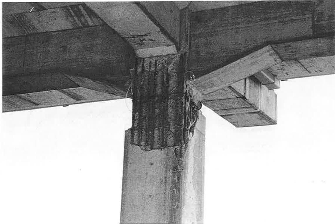
JRS-14. Column is damaged in both directions in addition to joint damage.
