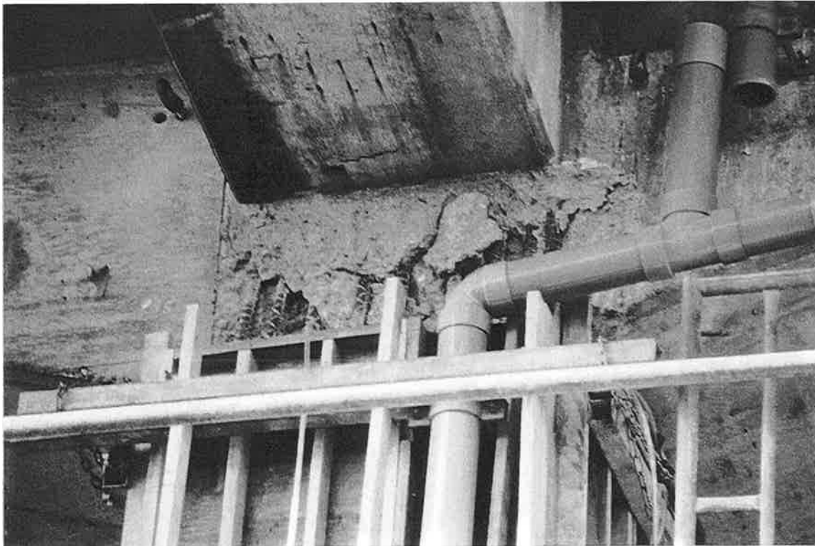
JRS-8. The cracking in this joint is limited to the zone below the confining catenary support beam at the top of the photo and the top of the column.
