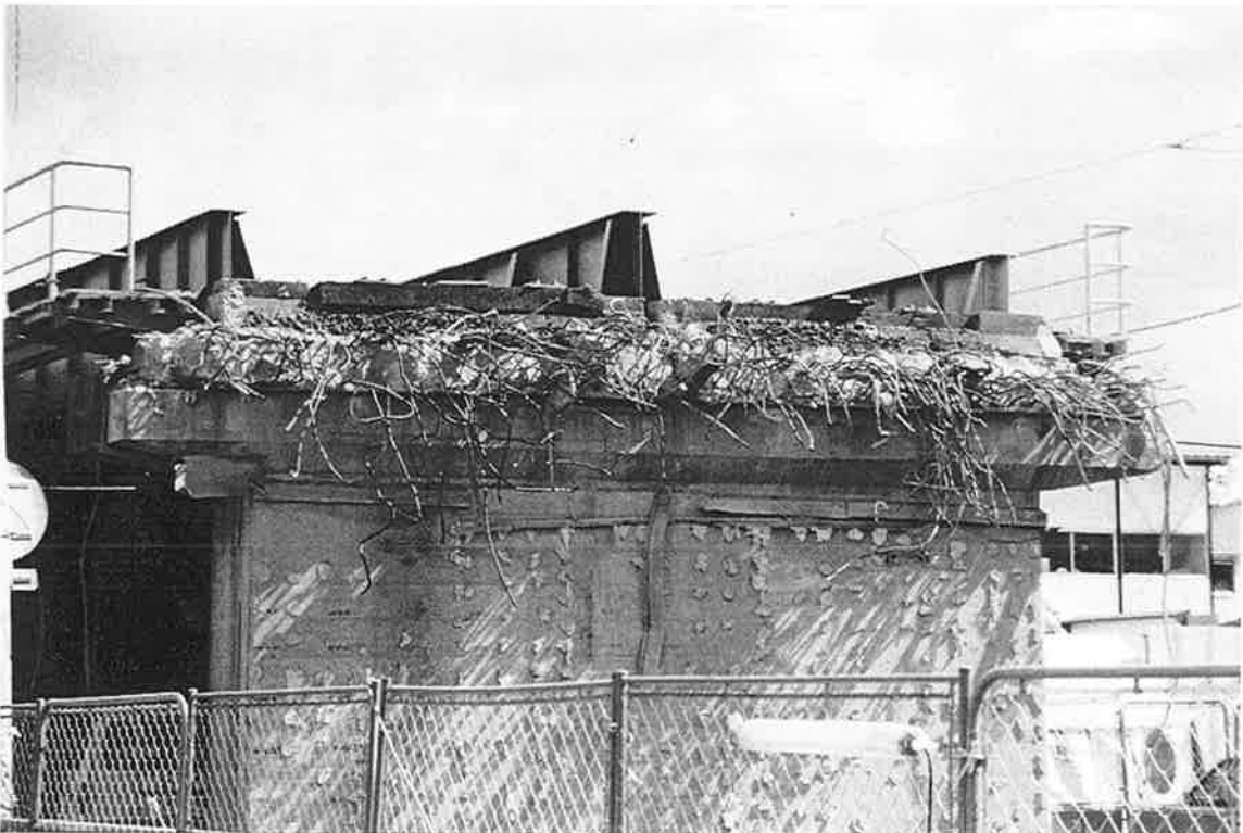
HC-7. Steel through girders at street crossing are the only remaining elements of the viaduct.
