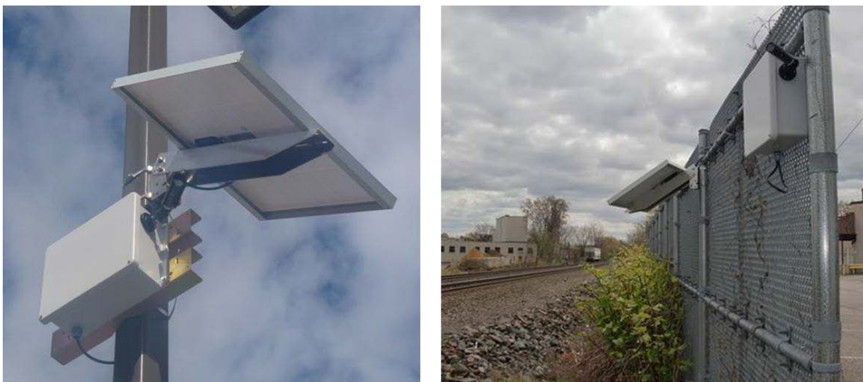
Figure 11. Solar Panel, Camera, and Box Housing the Digital Video Recorder
