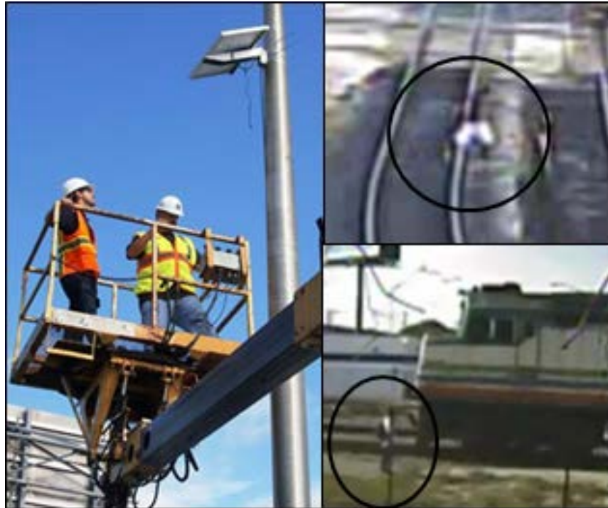
Figure 20. Data Collection System Installation for Targeted Data Collection (November 2012)
