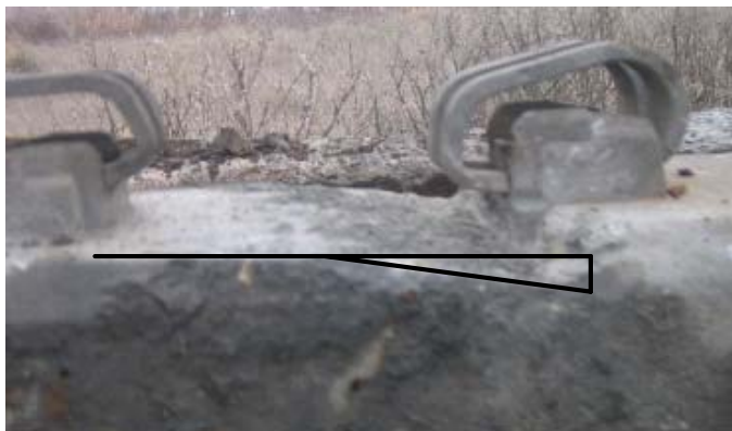
Figure 1. Triangular abrasion pattern in a concrete tie with black lines outlining a triangular pressure distribution assumed for this analysis.
