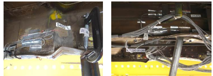
Figure 22. Buckling to Left Side Sill (Left) and Center Sill (Right) During Event 5
