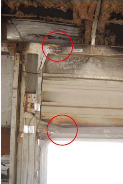
Figure 20. Damage to Cross-section 2 Left Roof and Upper Window Rails
