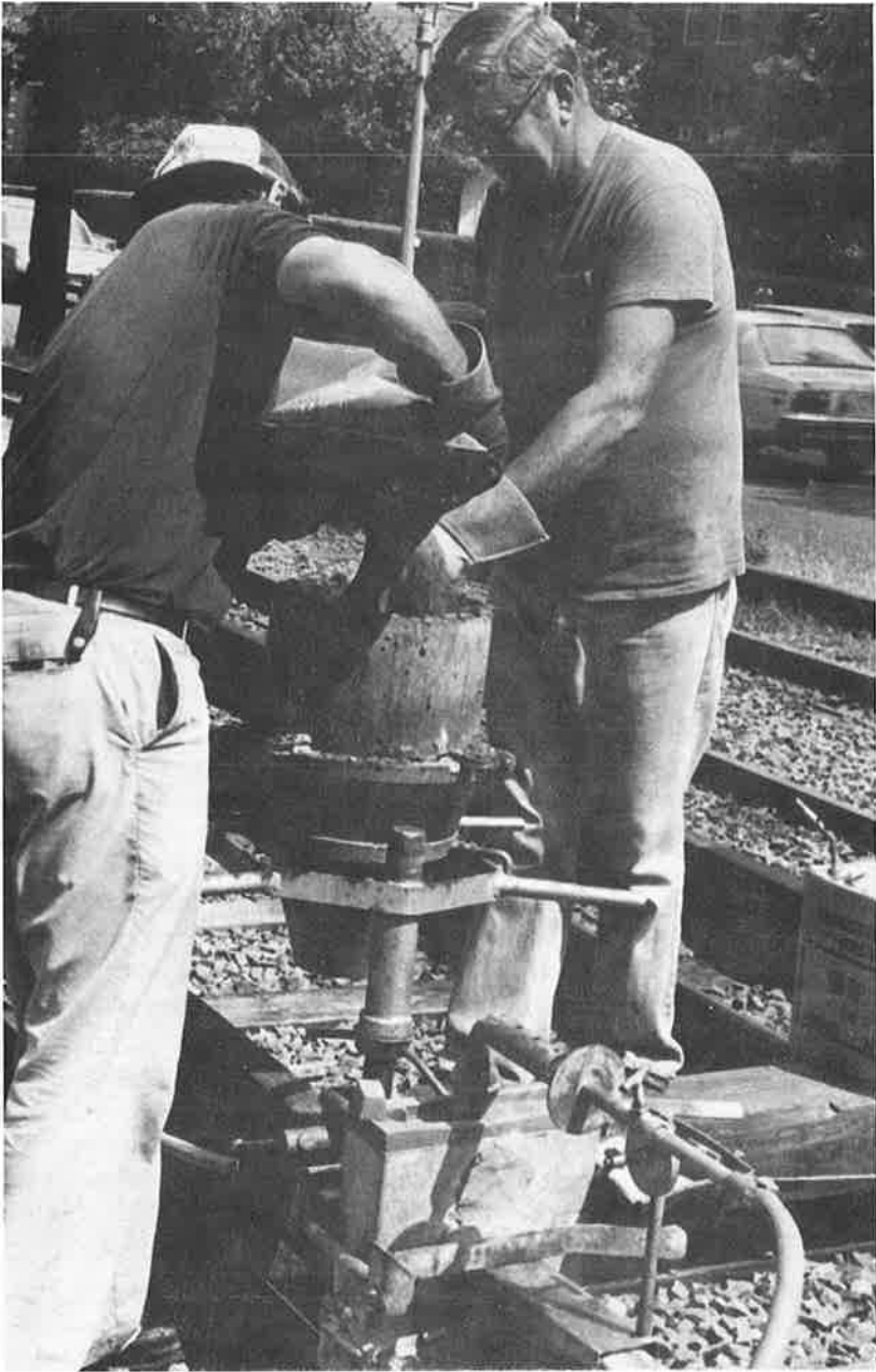
Thermite welding of transit track is becoming widely accepted. Various steps in the process are shown here.
