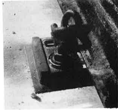
Direct fixation fasteners can usually be used to hold the rail, such as this elastic fastener.
