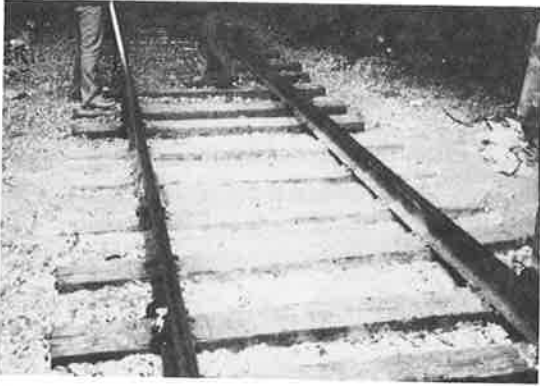
Timber ties showing signs of deterioration.
