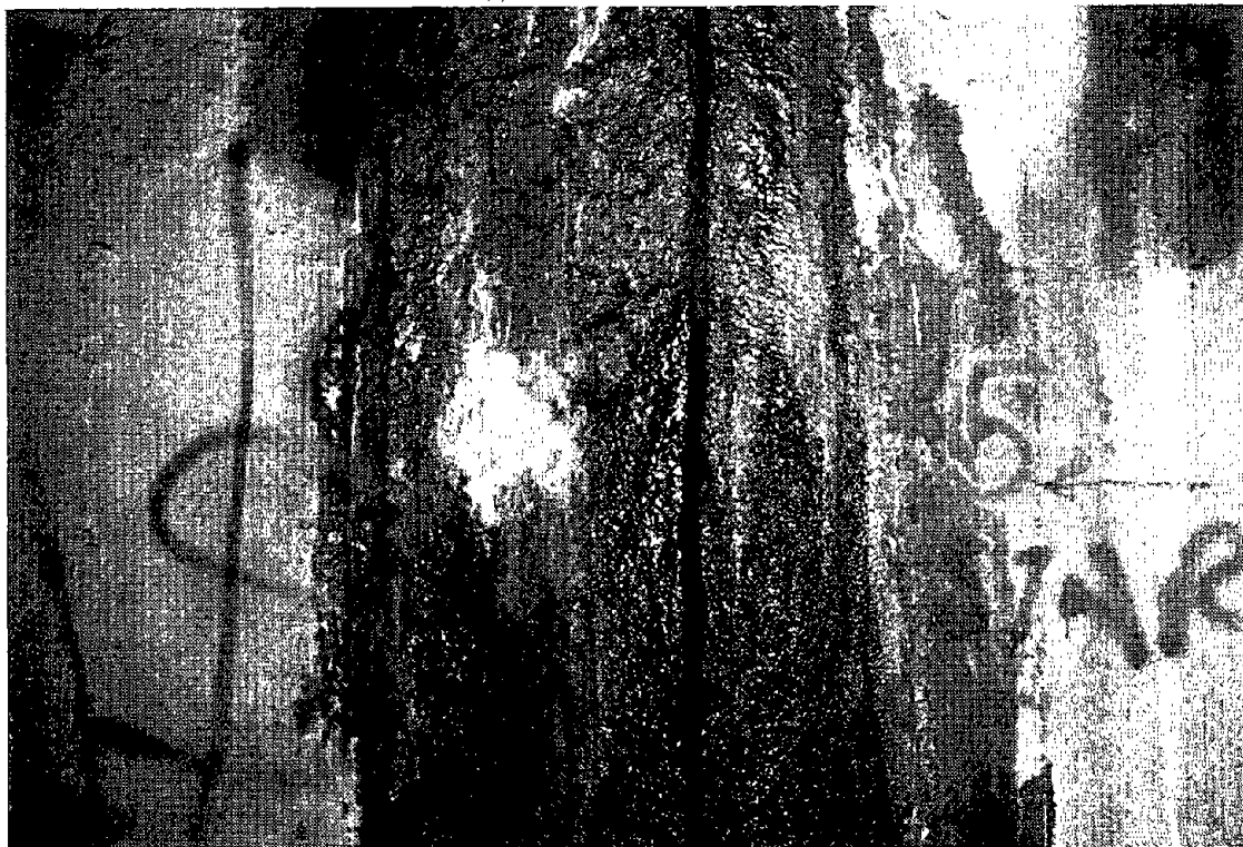
FIGURE 9.8 LEAKS THROUGH WALL JOINTS
