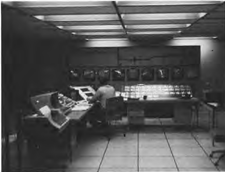
Figure B-3. Surveillance and Control Center, I-35W, Minneapolis, Minnesota
