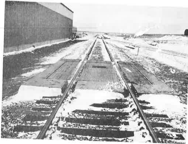
Figure 3-3 Track Scale Installed in North Leg of Wye Track Just North of the Transit Maintenance Building
