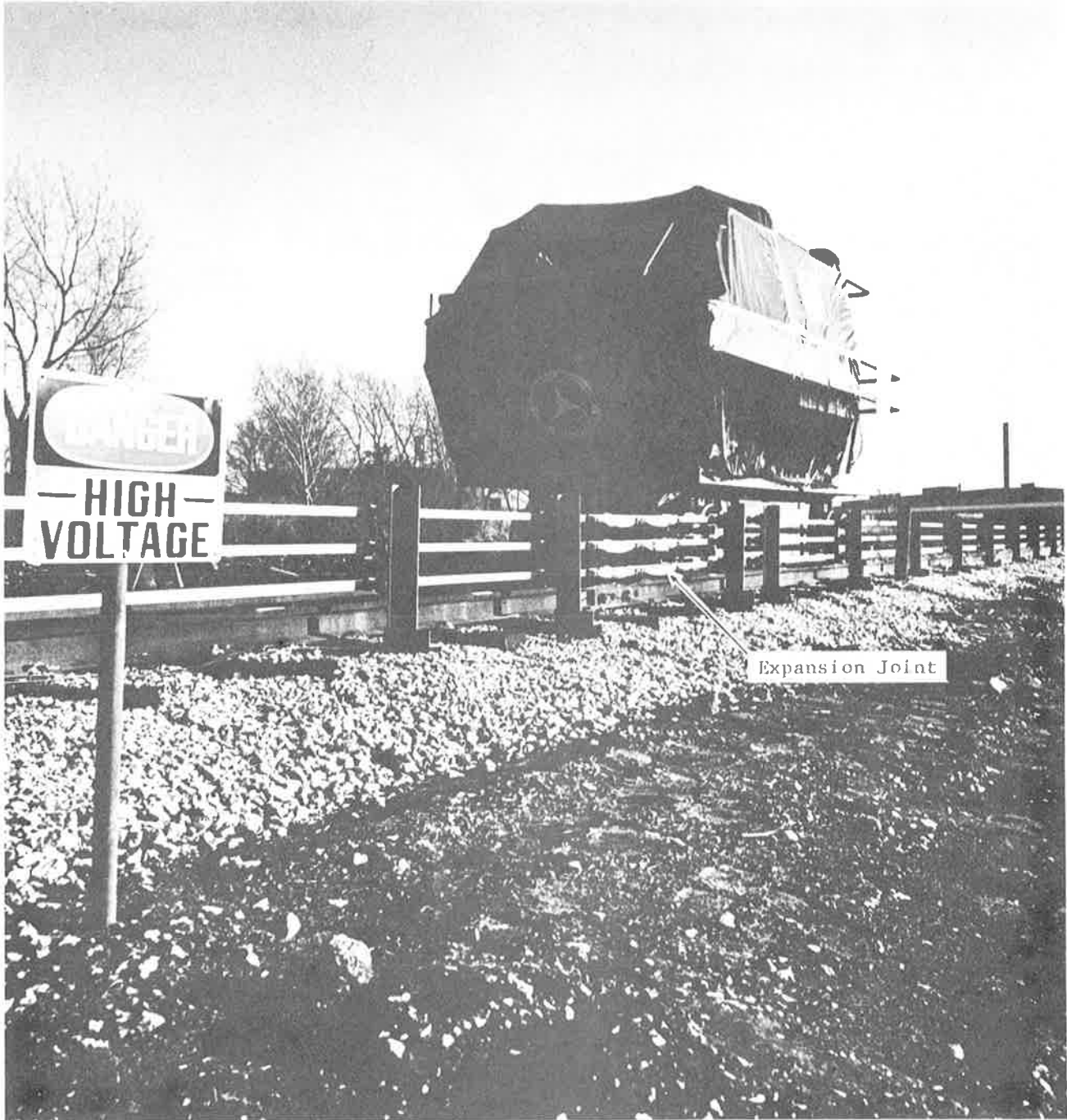
Expansion Joint - Power Rail
