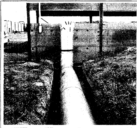
Figure 2-13. Blower Inlet Pipe
