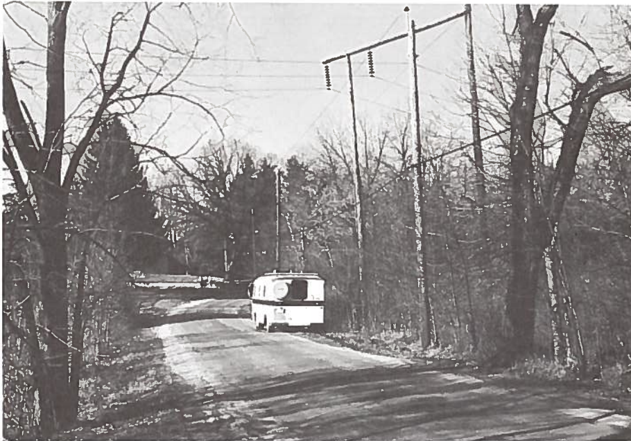
Figure 1-1. Typical 115 kV Power Line
